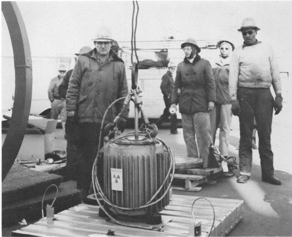
Fig. B-14. Generator Is Removed from Shipping Pallet (note gantry crane cables attached)
