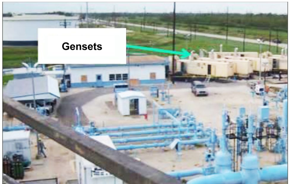
Figure 12: Colonial's Portable Generators
