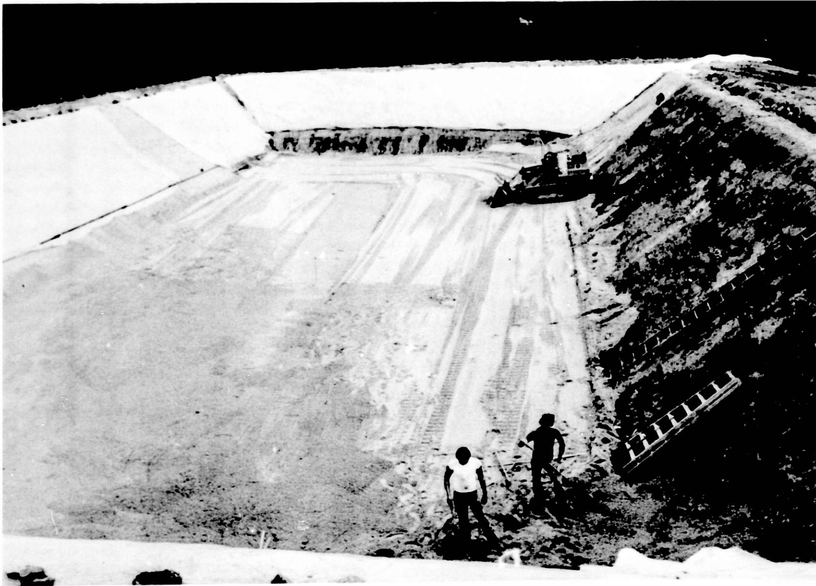
Fig. 11. Plastic Sheets on the Slopes of the Pond to Prevent Rain Erosion during Construction
