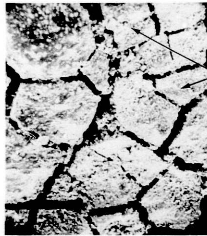
SURFACE EFFECTS OF EXPANSION DUE TO HYDRATION 330X
