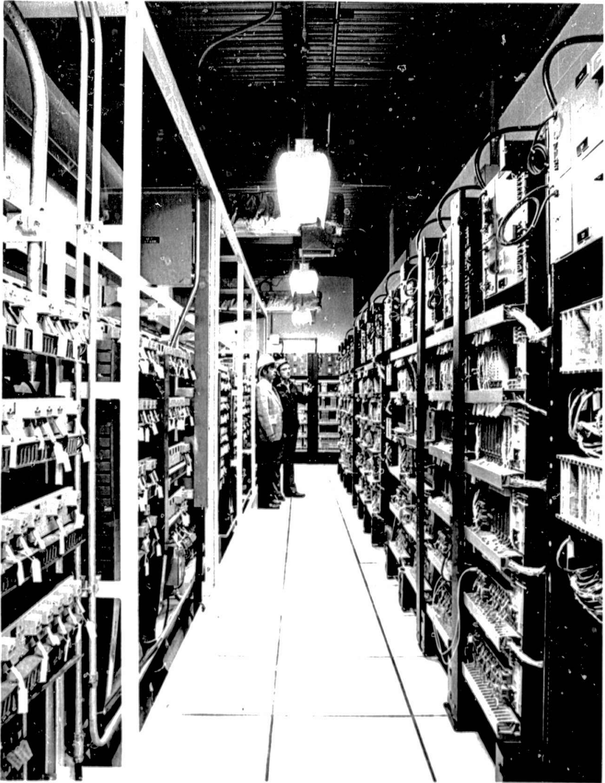
Fig. 6. Rear View of Instrumentation Panel
