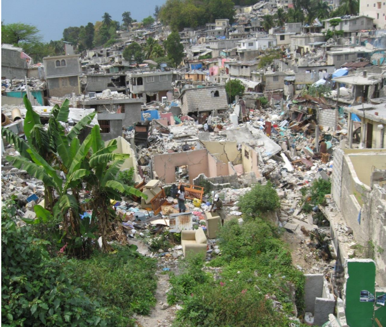
Figure 6. Destruction of civil structures by the earthquake in Port-au-Prince, Feb. 27, 2010. Photo by author.
