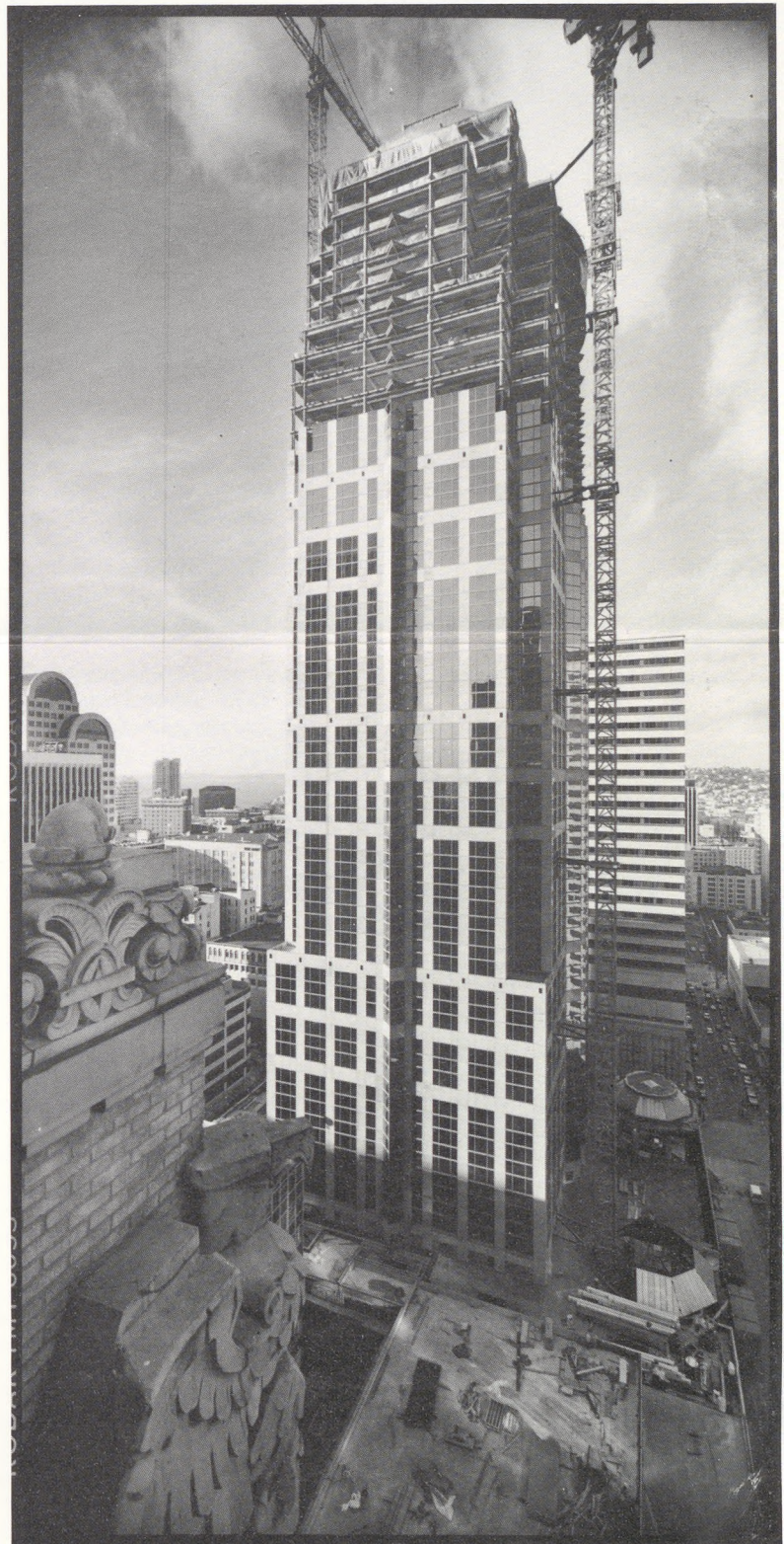
Pacific First Centre in Seattle was photographed by John Stamets with an ultra-wide "Skyscraper Camera"
