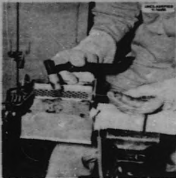
Fig. 6.10. Welding of a Header of the Intermediate Heat Exchanger No. 2. The strongbacks used to minimize distortion may be seen.
