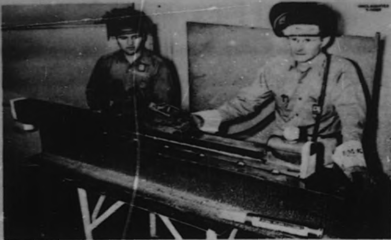
Fig. 6.14. Intermediate Heat Exchanger No. 2 After Completion of the Root Pass of the Pressure Shell Weld. Strongback used to minimize distortion.
