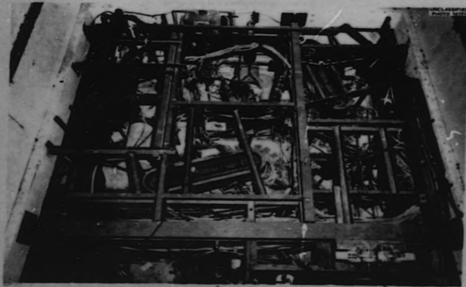
Fig. 6. Heat Exchanger Pit Showing Components of Fuel System Before Dismantling Operation.
