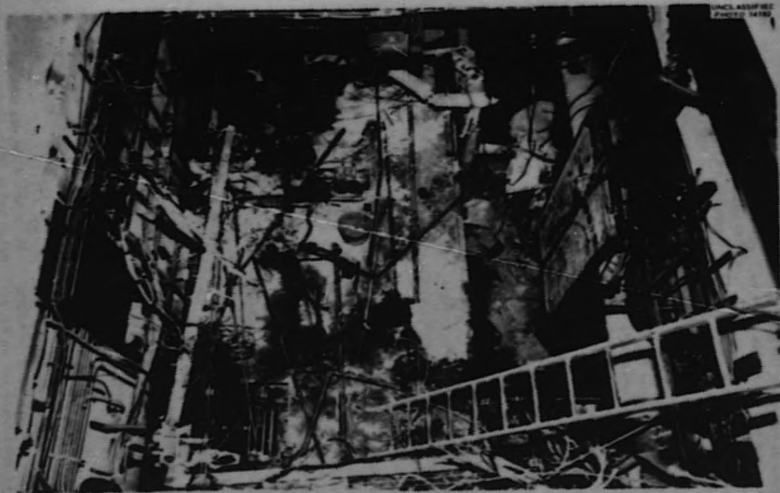
Fig. 5. Heat Exchanger Pit After Removal of Sodium System Pumps and Heat Exchangers and Lines. Note lead shield used to protect workers from fuel system radiation.
