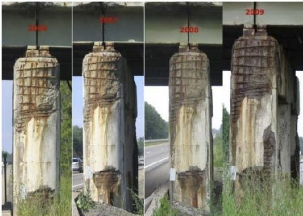
Figure 1.1: Corrosion in the bridge over the years [2]
