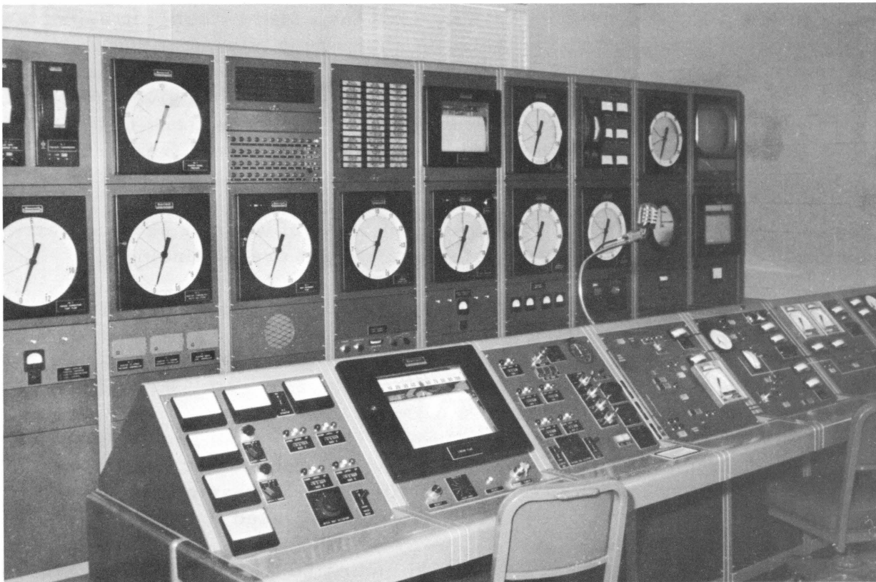
Fig. 27. Control Console and Recorder Panel
