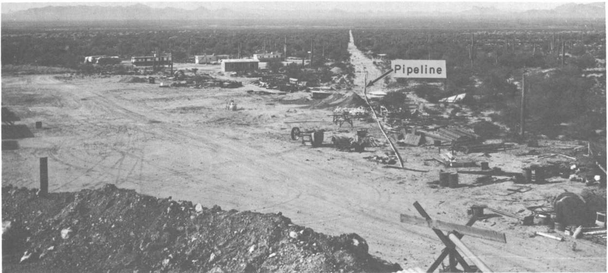
FIGURE 21. - Surface Pipeline and Trailer Camp, Lakeshore, Trans-Arizona Resources, Inc., Pinal County, Ariz.
