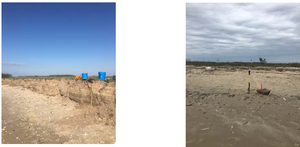
Figure 5.1: Scarp-like barrier in Zone 2 (left) and a sloping barrier in Zone 3(right).
