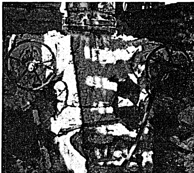
Figure 4. View of wellhead valves after shutdown.
