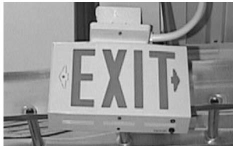
Figure 4-11 LED emergency exit sign
