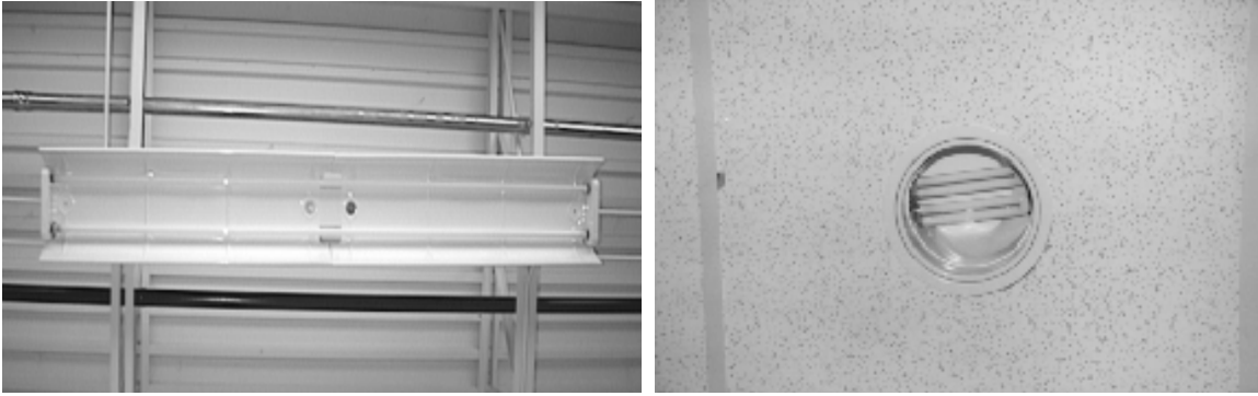
Figure 4-10 Efficient electric lighting luminaires include T-8 (left photo) and CFL can fixtures (right photo)
