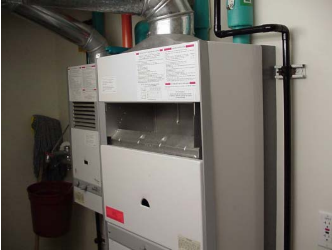
Figure 4-22 Tankless DHW heaters
