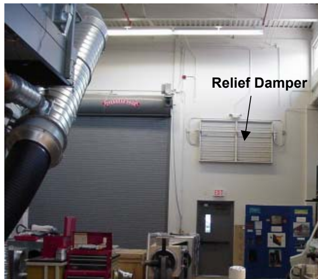
Figure 3-10 Relief damper location on east high-bay wall
