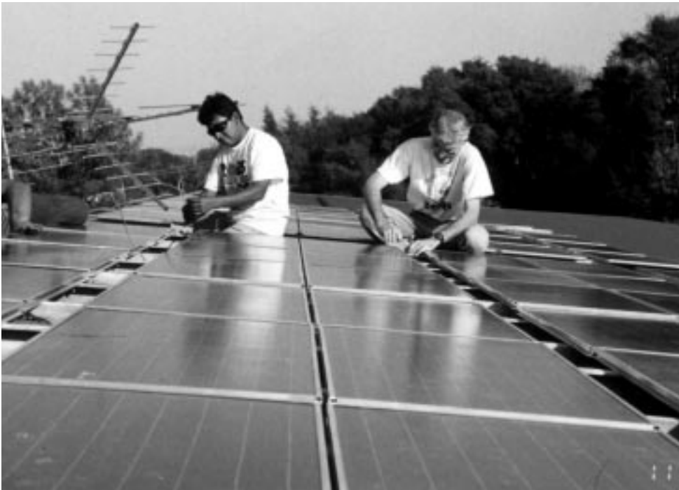
Workers install an 8-kilowatt PV system on the roof of Western Area Power Administration's operations center in Folsom, California.
