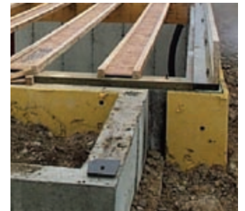
Extend exterior insulation all the way to the sill where permitted by code. (Source: CARB)
