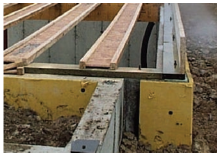
One recommendation was to extend exterior foundation insulation all the way to the sill rather than cutting it off at ground level.
