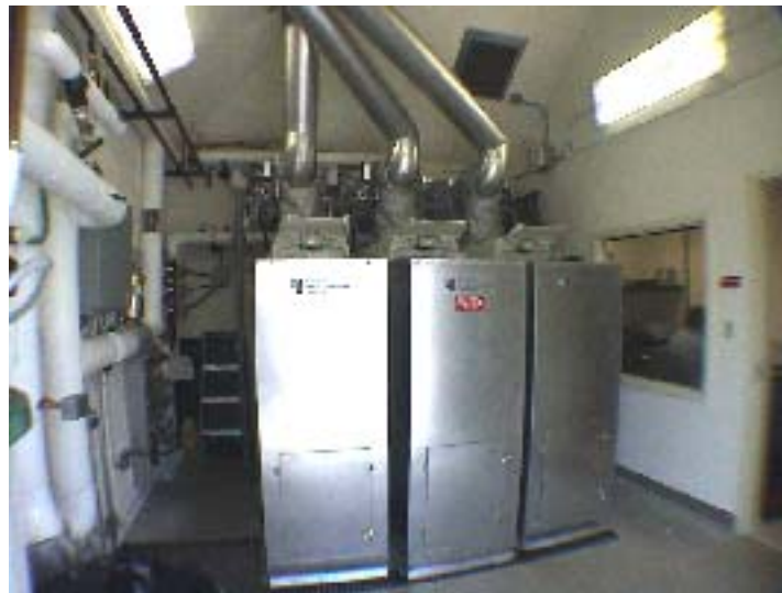
Figure 4: CHP Test System Building
