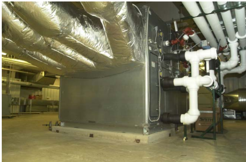
Figure 99. Existing heating system
