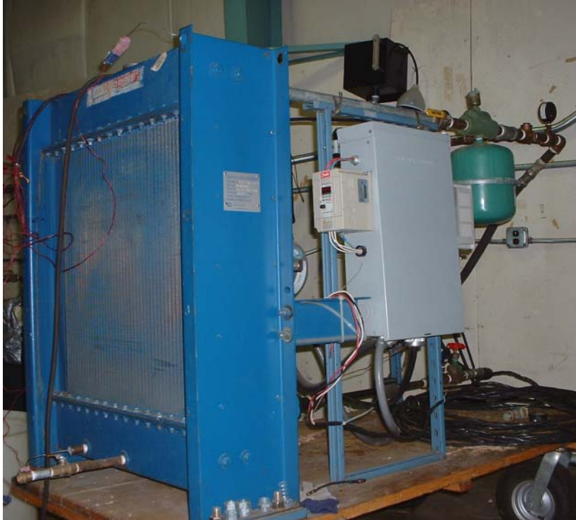
Figure 71. Heating heat exchanger for warehouse with instrumentation
