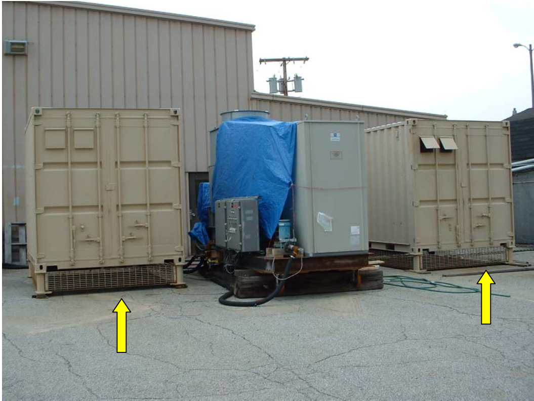
Figure 28. Two packaged CHP systems (Boxes on either side of the absorption chiller skid)
