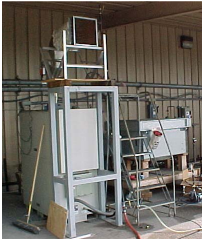
Figure 72. Microturbine and heat exchanger for warehouse
