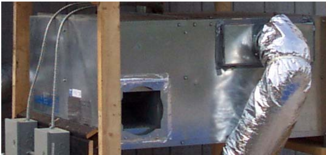
Figure 33. Energy recovery vent
