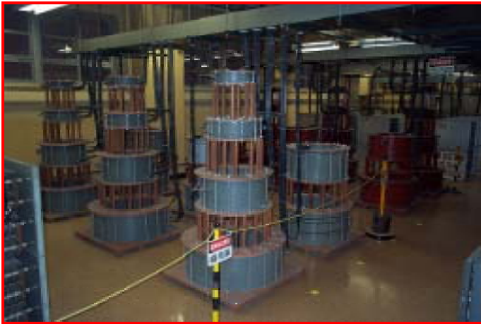
Inductive load banks UL uses for anti-islanding tests at the Northgate, Illinois, facility
