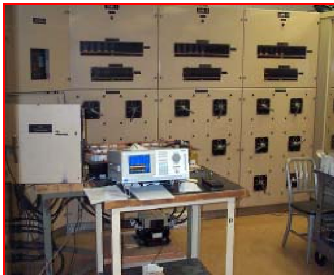
Three-phase anti-islanding test equipment at UL
