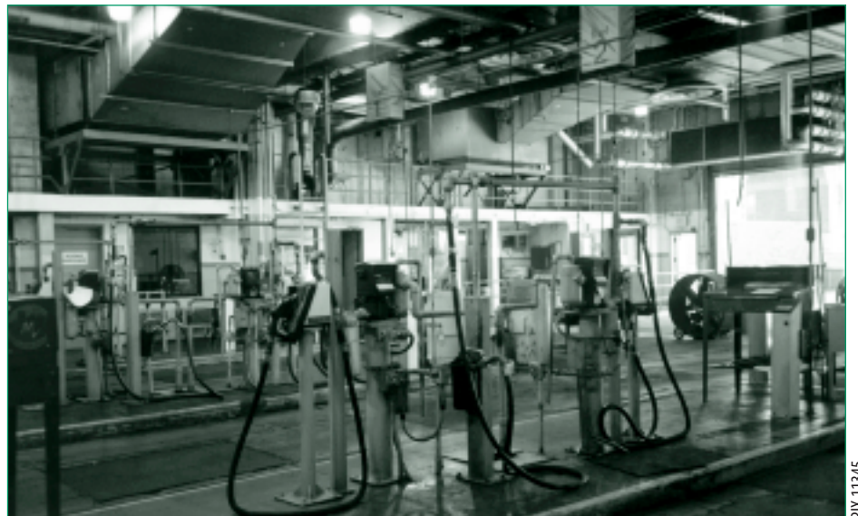
Figure 4. Diesel fueling lanes at Manhattanville Depot
