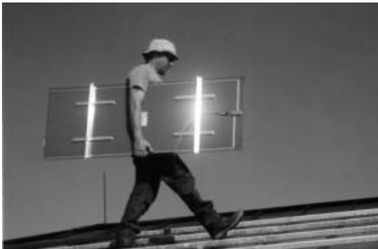
Worker transporting each BP Solar cadmium telluride module to the final site.
