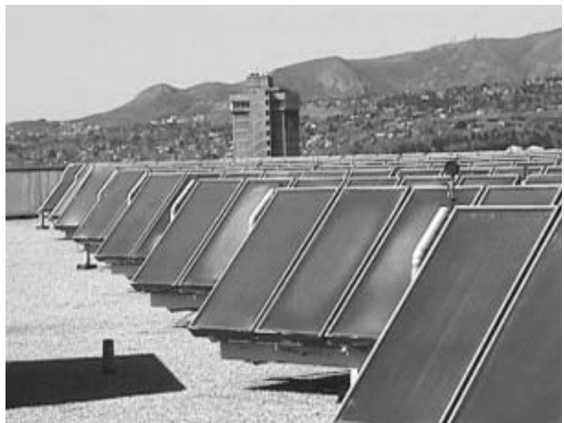
Solar Hot Water System at Salt Lake City Veterans Administration (VA) Hospital.
