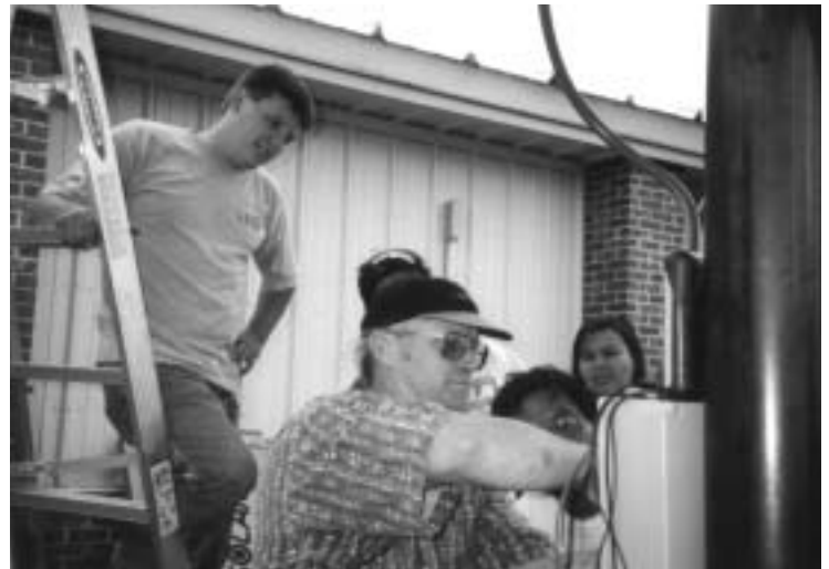
Field instruction in wiring a junction box by Kerry Kalarney, Sundance Solar
