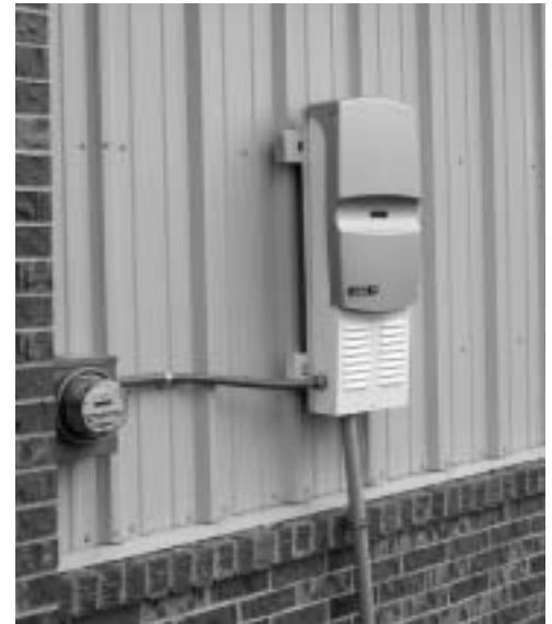
Inverter feeding AC electricity into building power supply and connected to utility meter.
