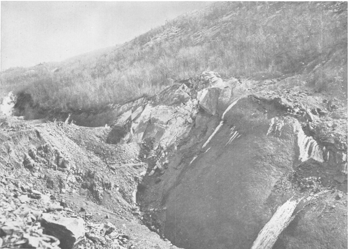
FIGURE 6.—Typical View of Stripped Bed at Outcrop, Showing Lack of Provision to Keep Surface Water From Entering Mines.
