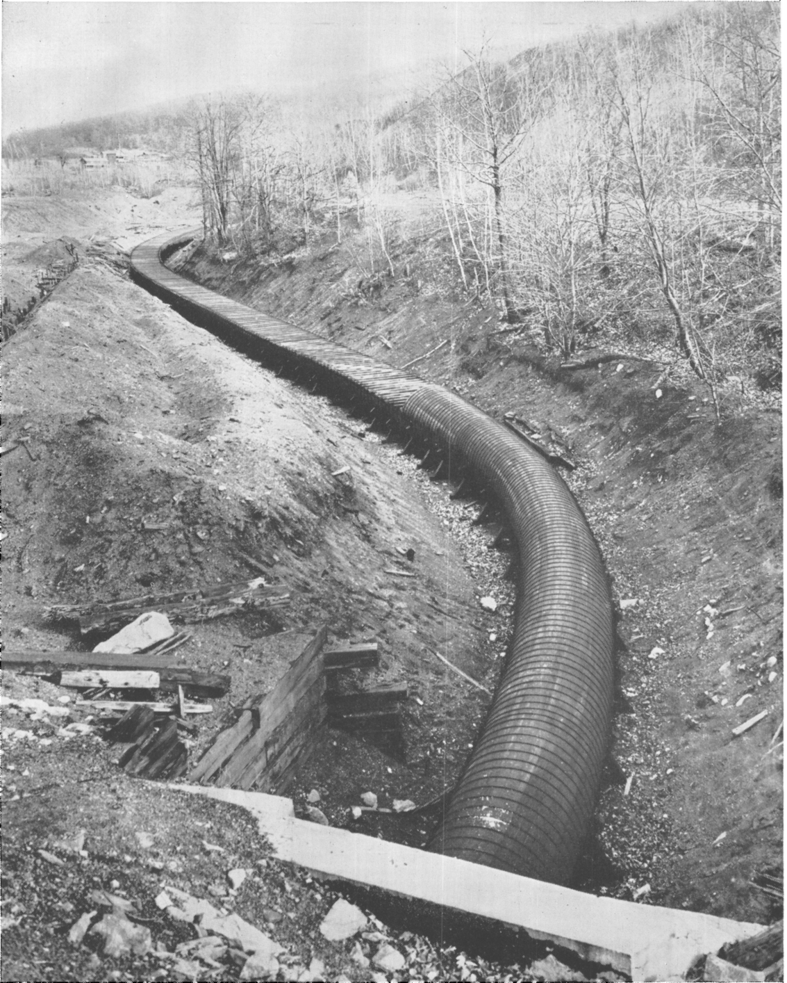
FIGURE 9.—96-Inch, Creosoted, Wooden-Stave Pipe Reduced to Semicircular Wooden-Stave Flume of Same Diameter.
