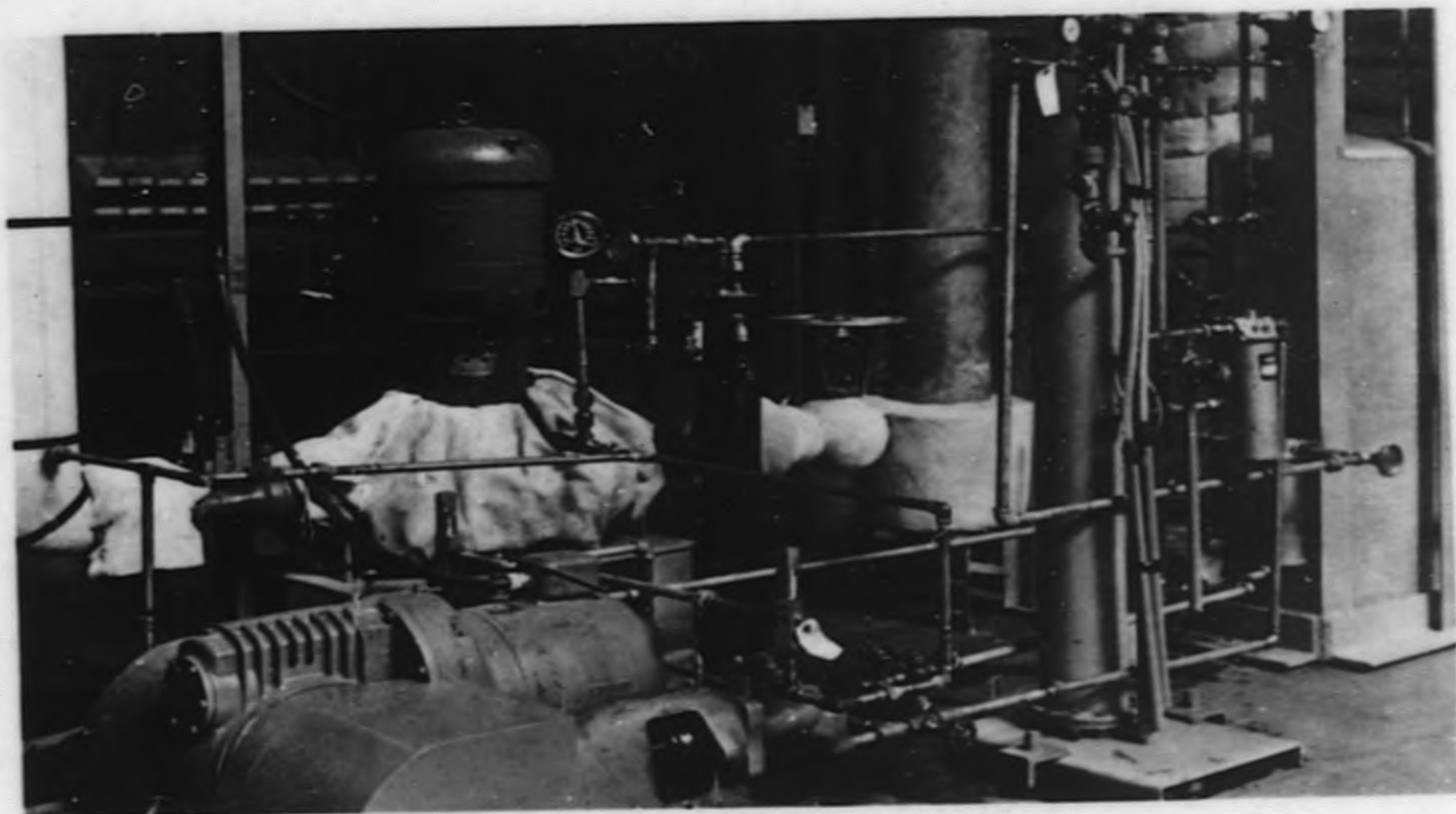
ORNL Test Rig - Select View of Piping #1
