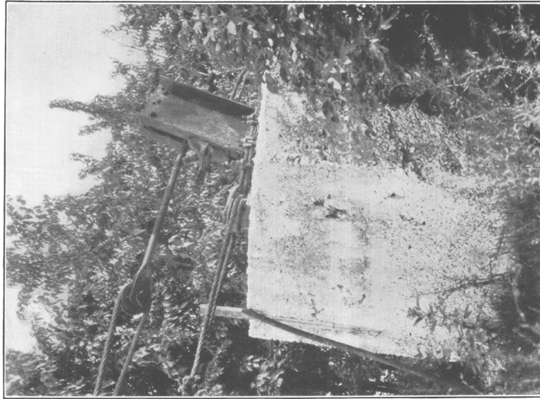
42. AN ANGLE STEEL AND CONCRETE GUY ANCHOR USED IN A QUARRY AT GANTTS QUARRY, ALA.
