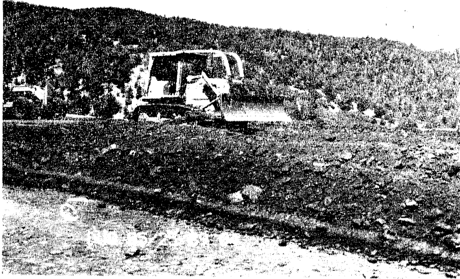
Preparing the disposal cell embankment at Bodo Canyon, CO disposal site for placement of contaminated material from Durango, CO, processing site.
