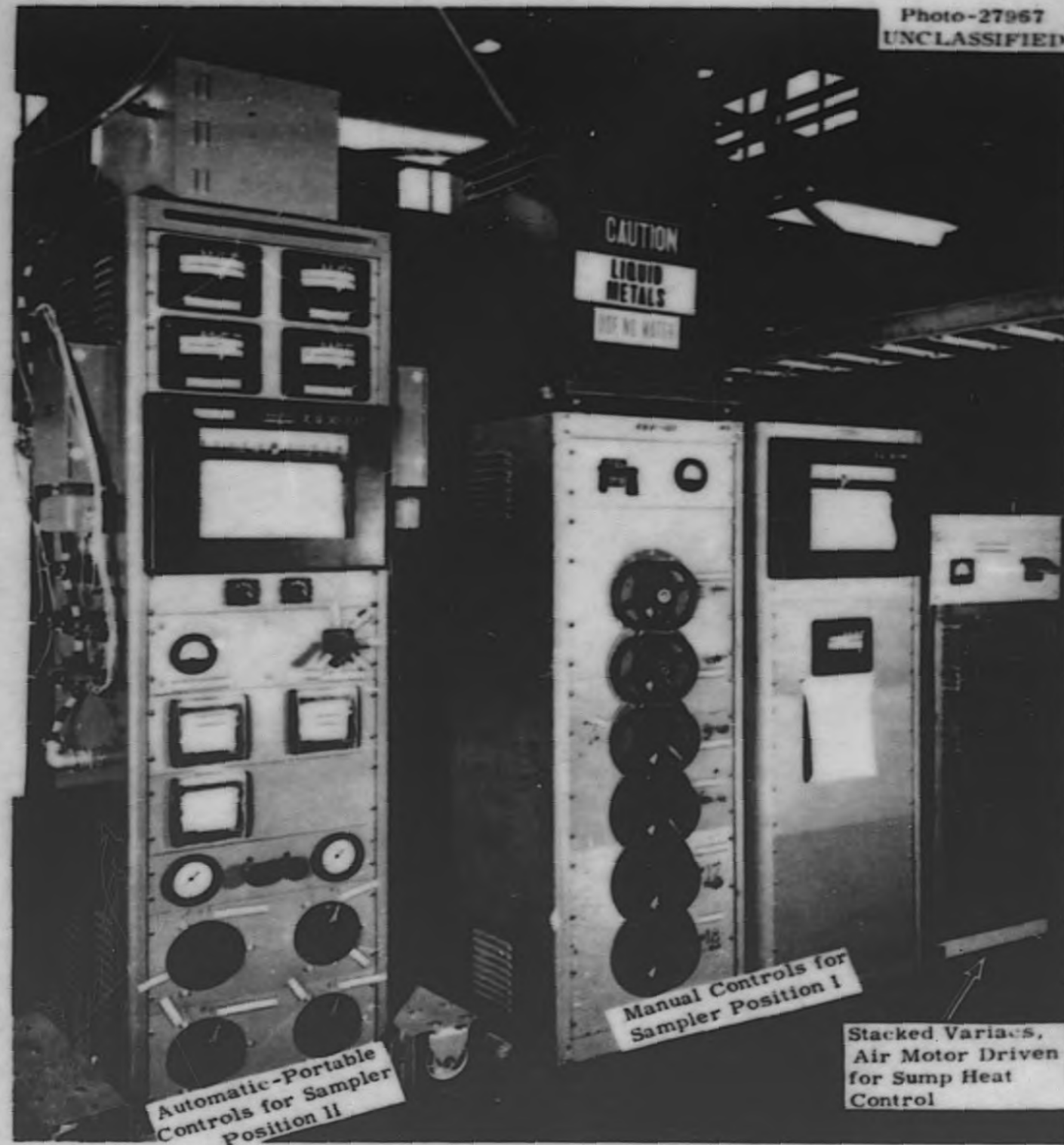
Figure 9 Instrumentation for Argonne Sampler Units Cold Trap Stand 1
