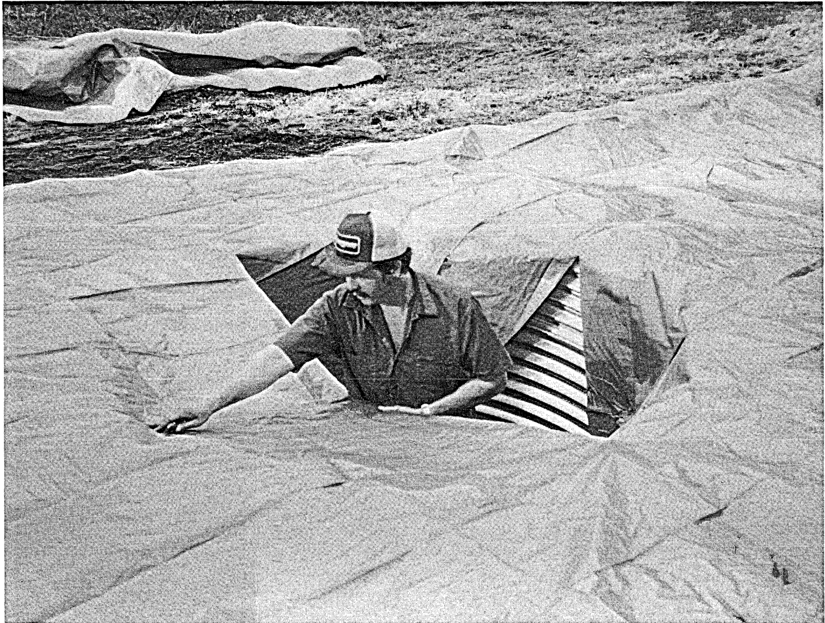
Fig. 9. Installation of ground protection tarpaulin at VC-1. Note the corrugated metal pipe cellar.
