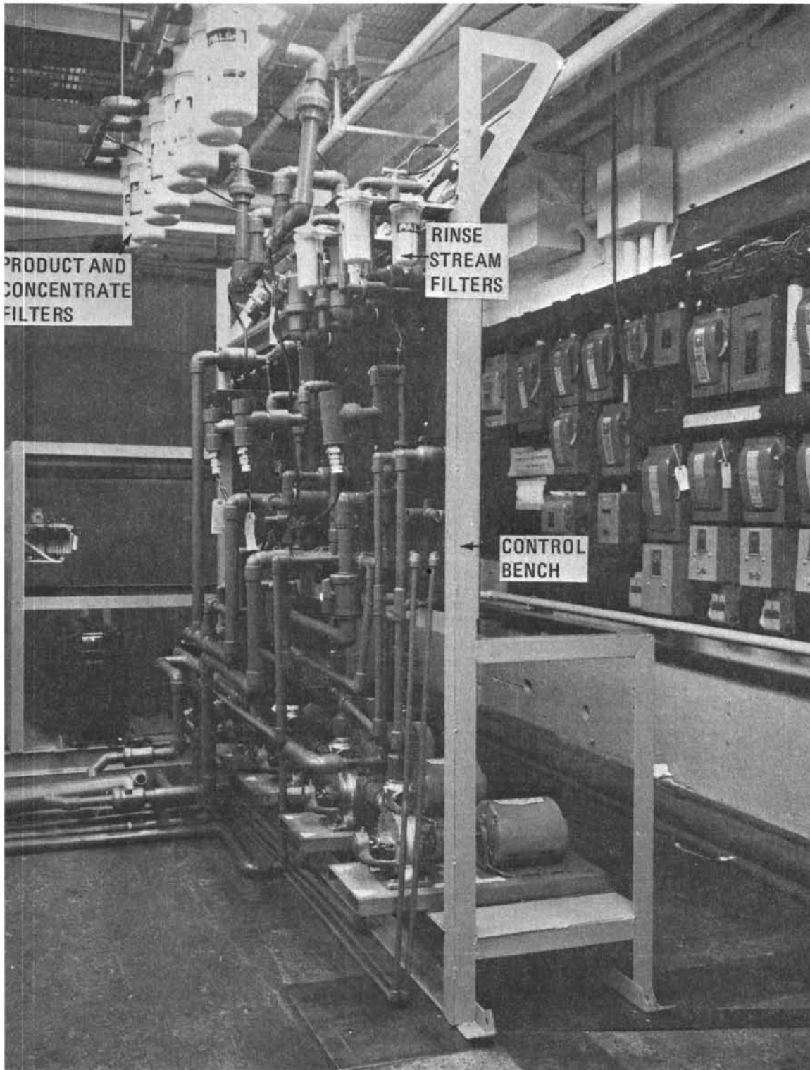
Figure 58 Operator's Stand of Pilot-Plant System X-29229
