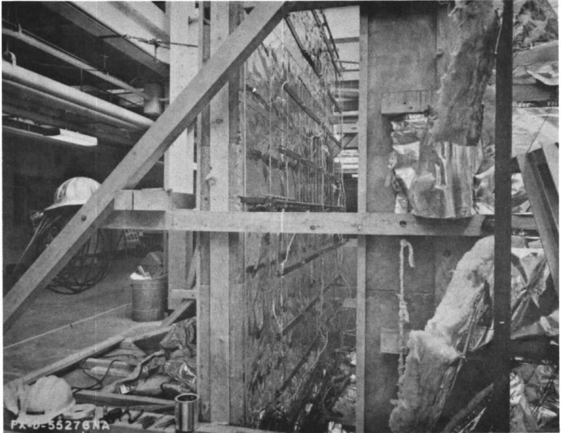
Figure IV-9. View of horizontal arrangement of strip heaters which supply the heat energy during testing. Photo PX-D-55276 NA
