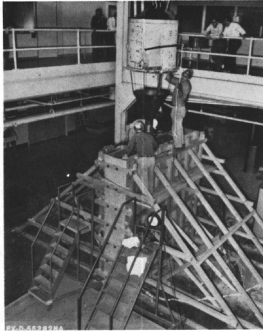
Figure IV-6. View of the forming and bracing during concrete placement. Photo PX-D-55282 NA
