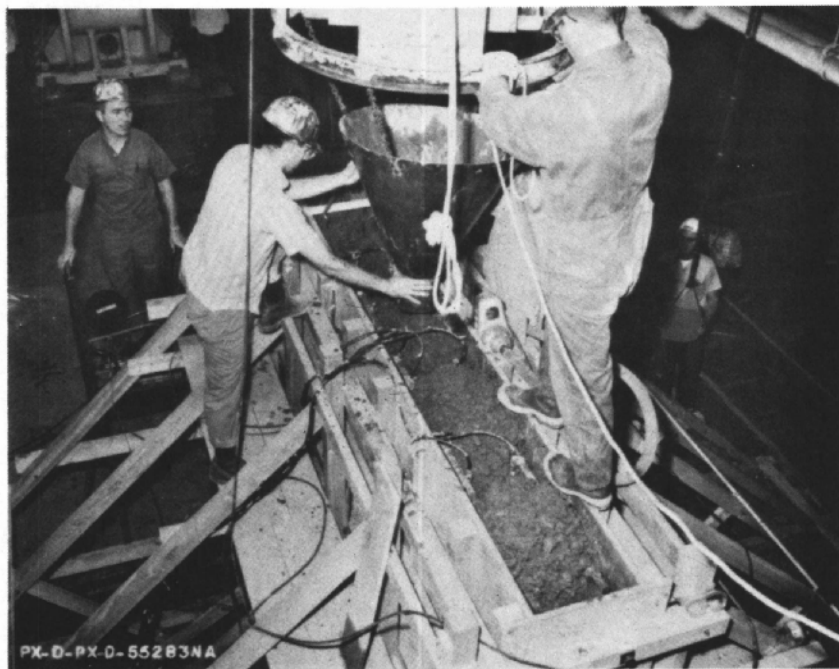
Figure IV-7. View during the latter stages of the concrete placement operation. Photo PX-D-55283 NA
