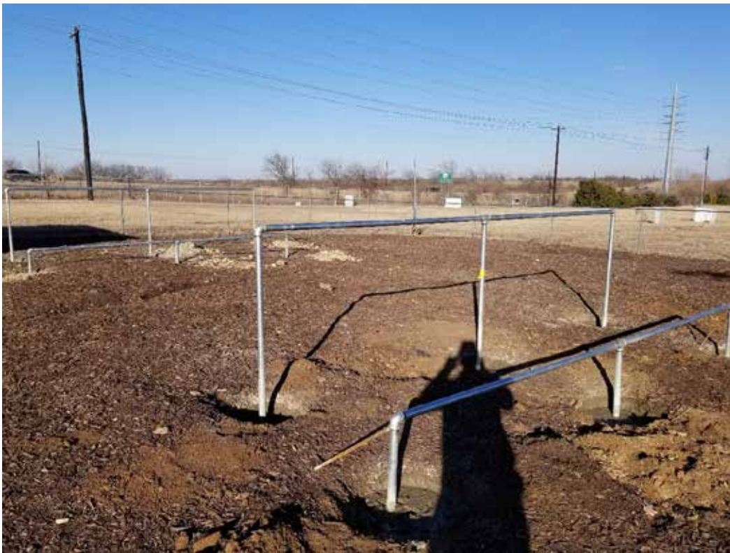
Figure 3.4 : Solar panel mounts
