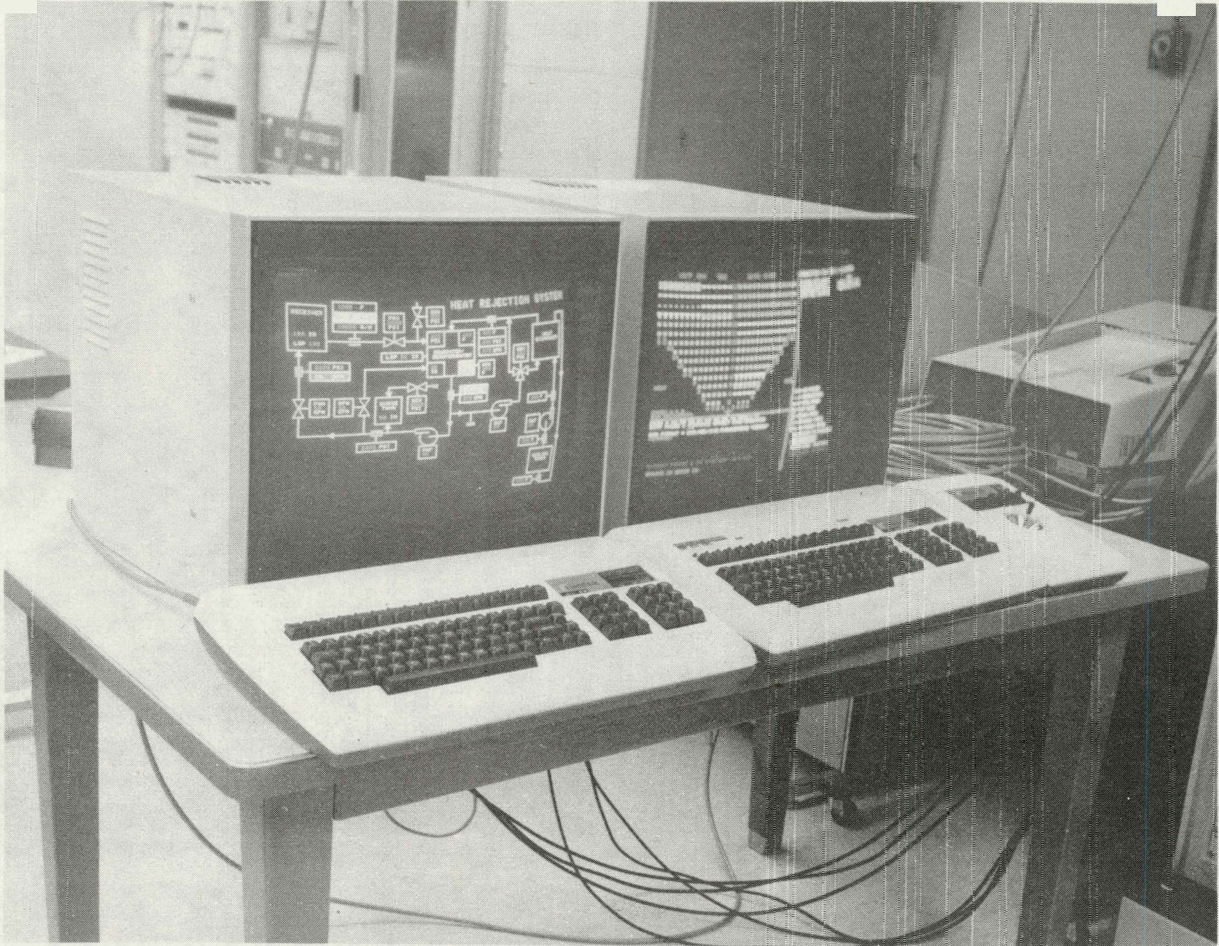
STTF CONTROL ROOM OPERATOR CONSOLE
