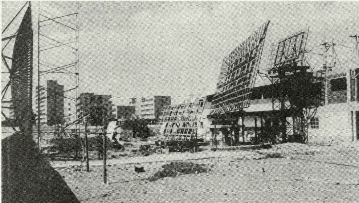
Figure 33. Construction of Solar Furnace Test Facility at National Research Center, Cairo, Egypt.
