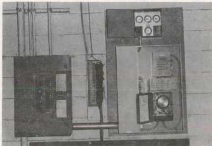
a - Timed Lights Control Panel Installation (Open)
