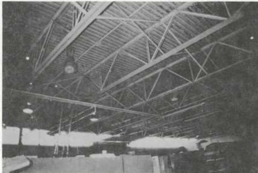
d - Typical Mercury Vapor Lamp Fixture Array
