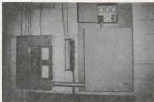
b - Timed Lights Control Panel (Closed)
