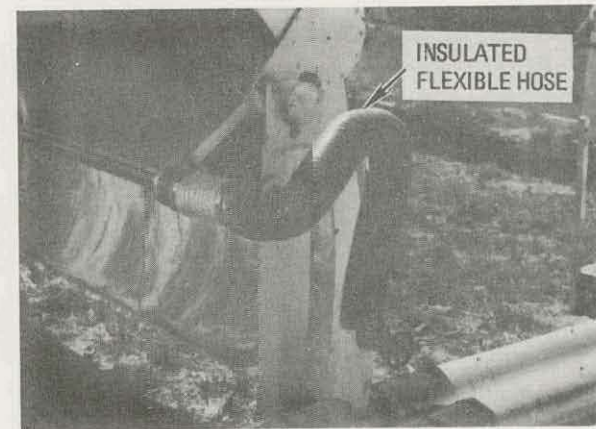
D. END OF ACUREX COLLECTOR STRING
