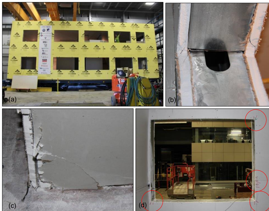
Figure 15: (a) Phase 2e specimen post-test (b) drywall cracking at interior window corner (c) drywall cracking and crushing at interior partition wall base (d) drywall cracking at interior window corners (location of cracks are encircled)
