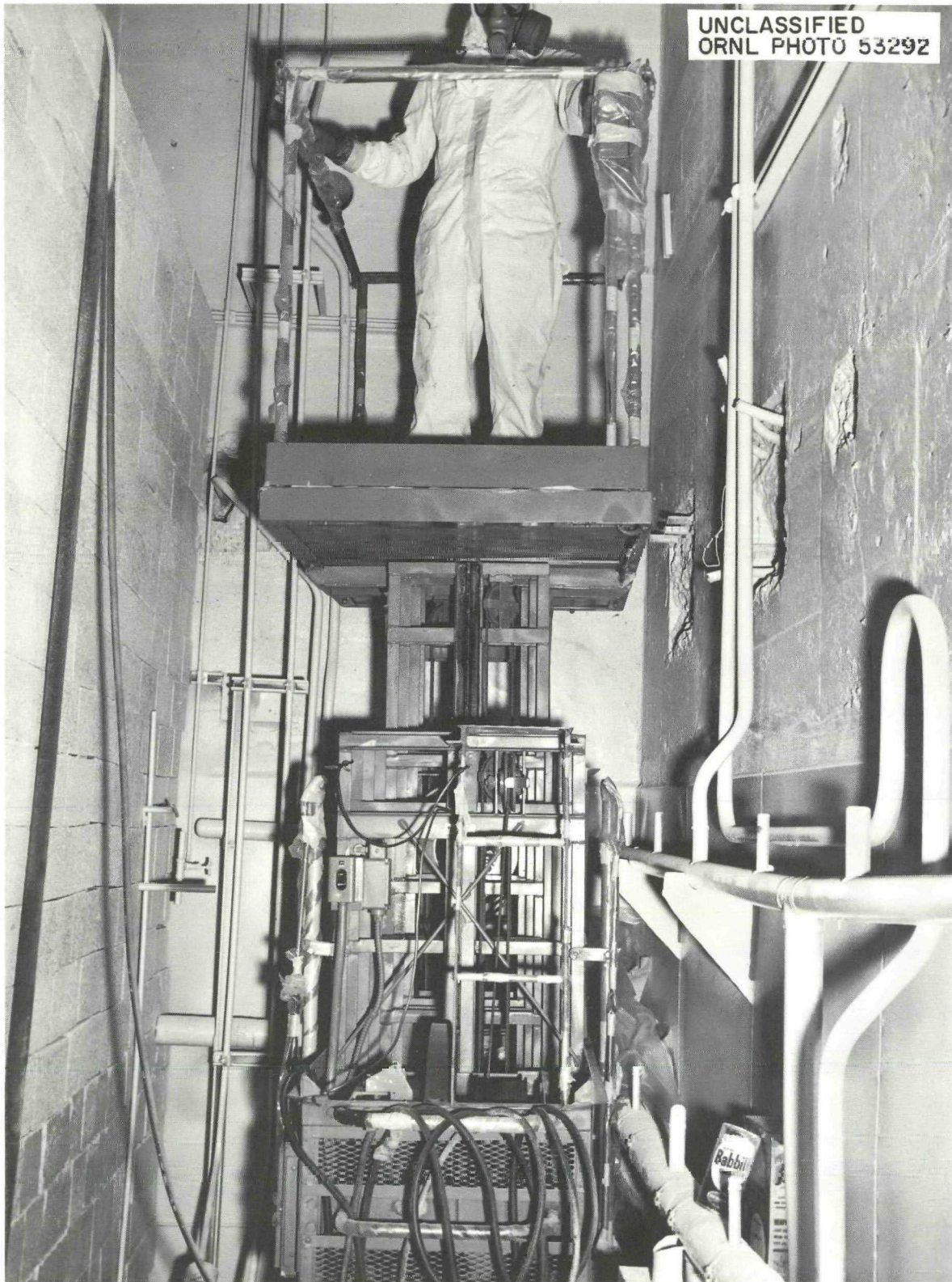
Fig. 5.3. Telescoping elevator used for removing shielding blocks.
