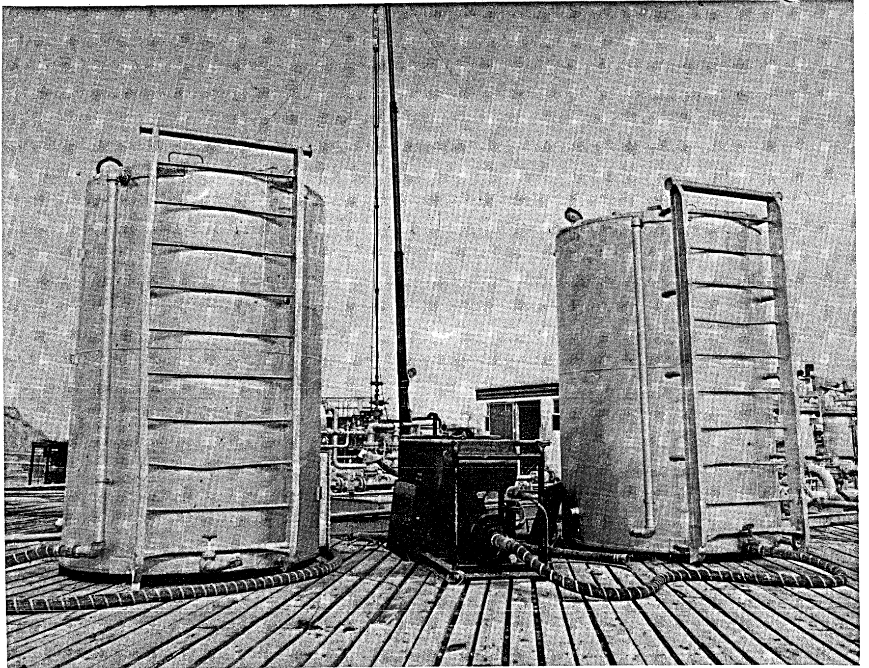
Photo 9-7 Pump and two 110-barrel tanks were used to calibrate the turbine meters.
