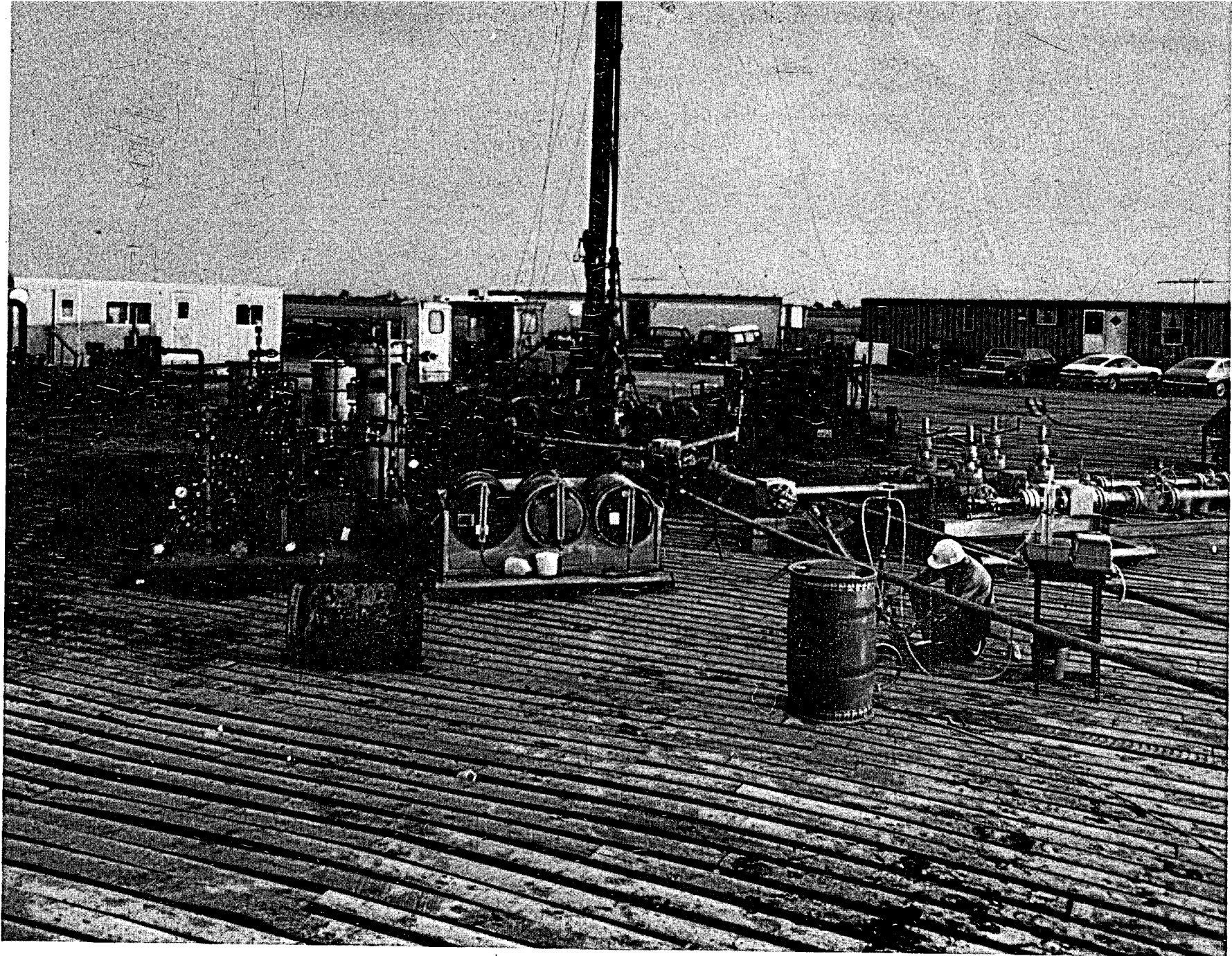
Photo 9-2 The unit with three chemical drums includes two high-pressure chemical inhibitor injection pumps.
