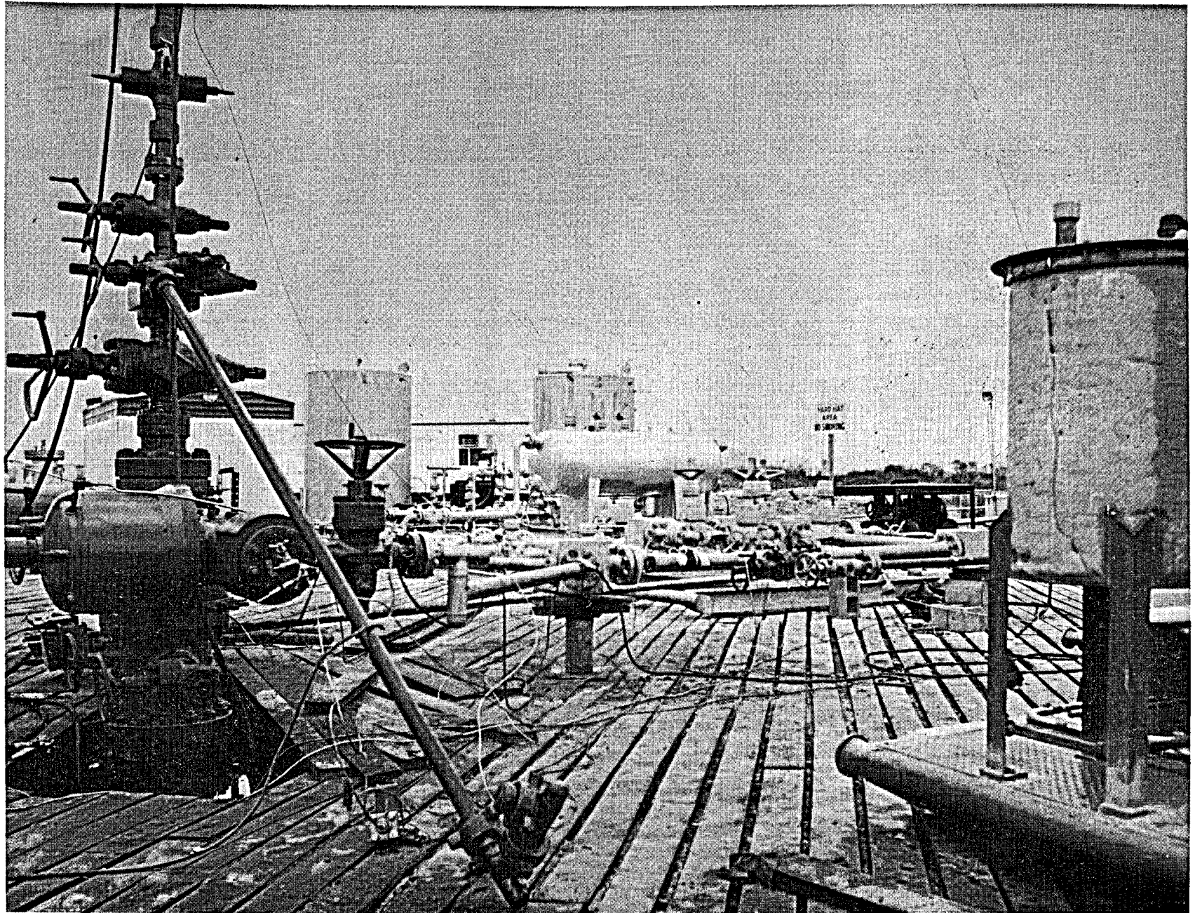
Photo 6-6 Note kill line connected to tubing wing valve on Christmas tree.
