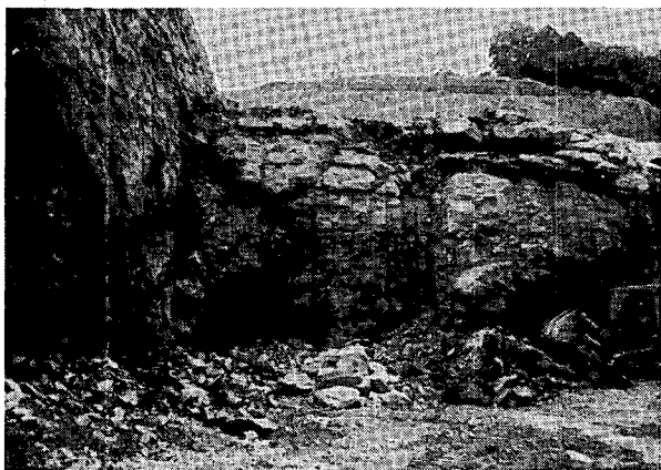
Fig. 5. Sheet joint in Upper Gilbert sandstone (to right of center), PB-6B.
