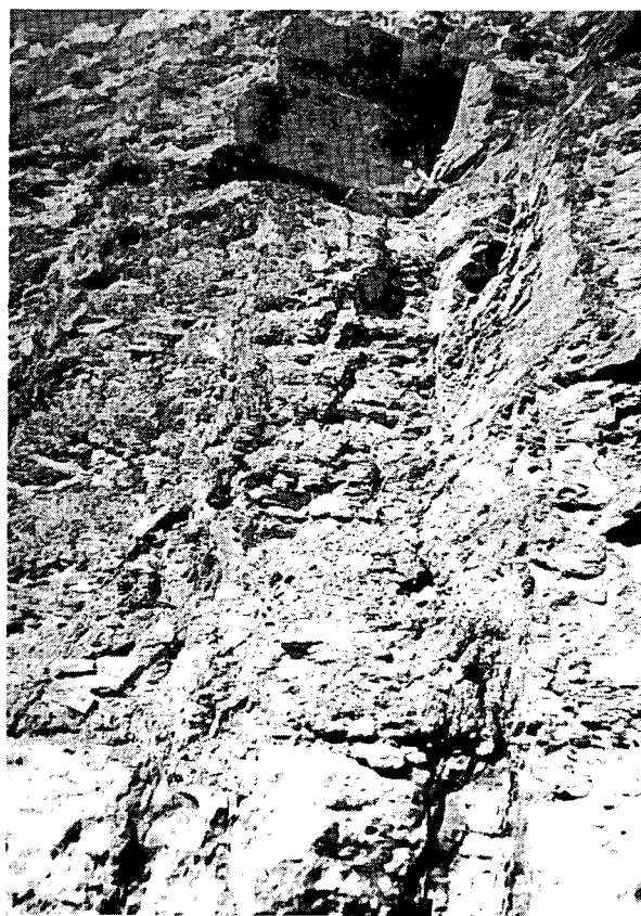
Fig. 4. Weathered sheet joint in fissile clayey shale, PB-3 (metal rule in lower left is 2 in. square).
