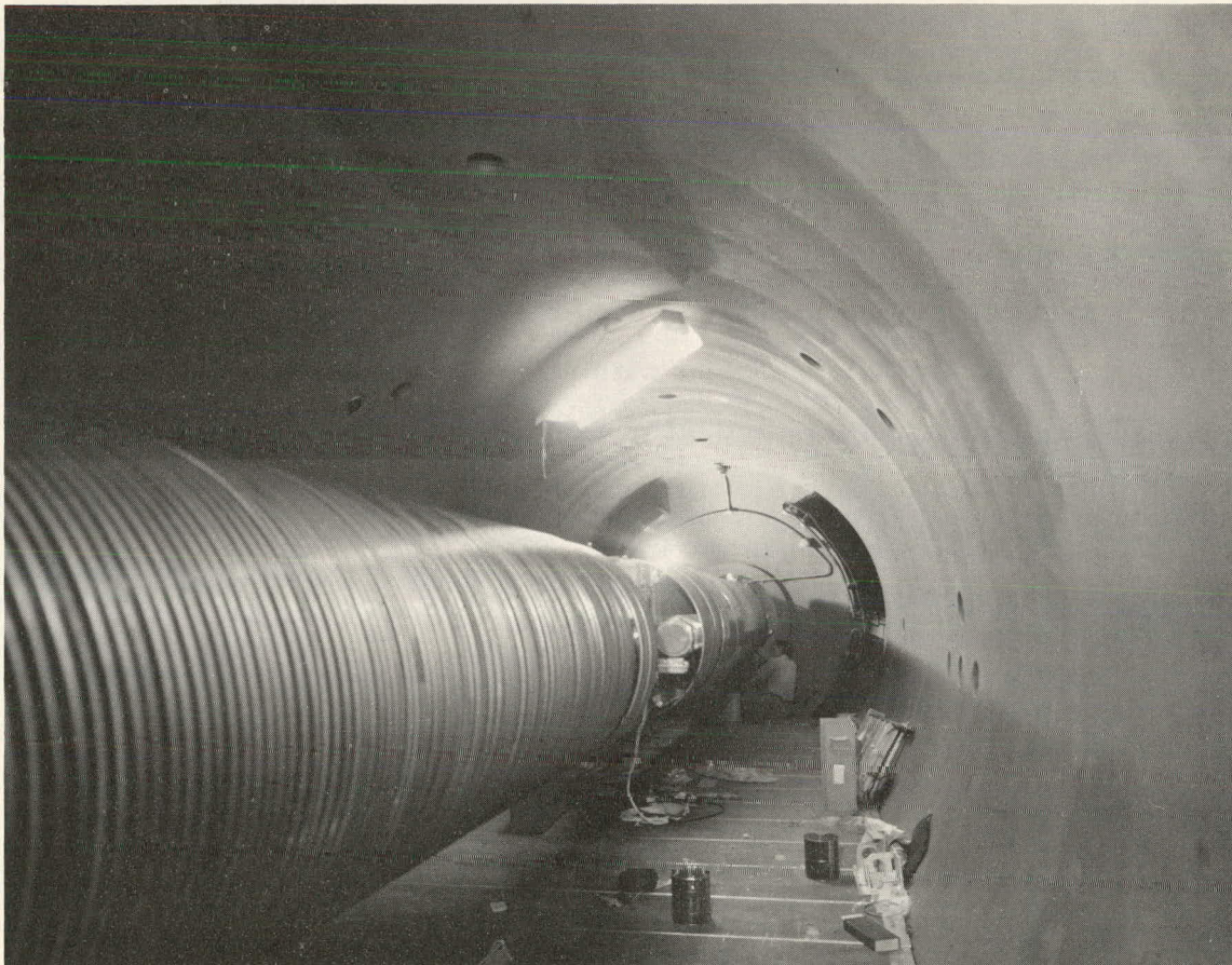
Fig. 2. Installation of the new FN tandem. The two small pictures at the top show the tank being moved into the vault on 2 July 1967. The larger picture below shows the high-voltage structure inside the tank as it looked on 21 July 1967 when its assembly was almost completed.
