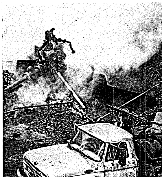
Figure 5. Steam well blowout at the Geysers Field, California. Illustrates the need for precautions to prevent blowouts from occurring even at producing fields.
