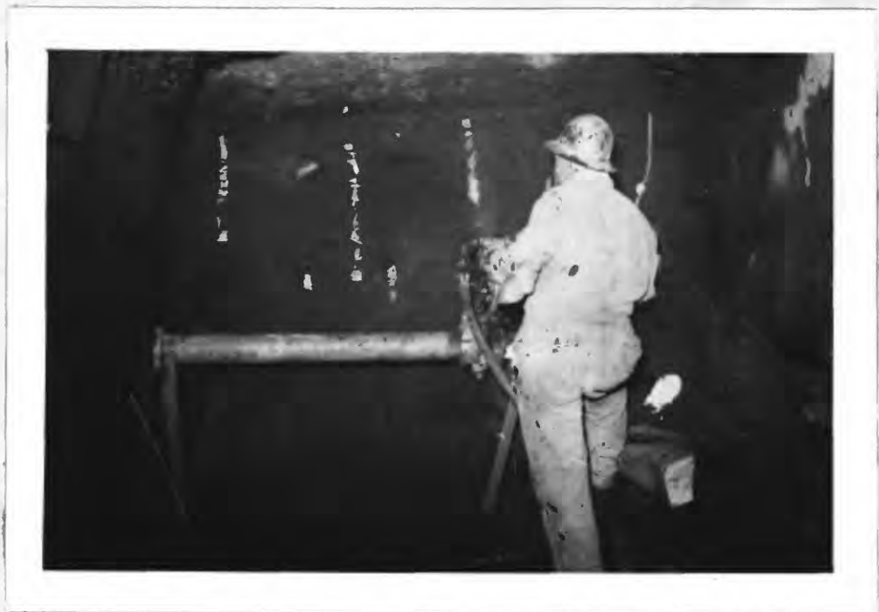
Fig. 6. Face of adit at 58.5 feet, showing drifter, bar, and supports. White paint lines show locations of lines of holes. Note joint face on left. January 24, 1949.
