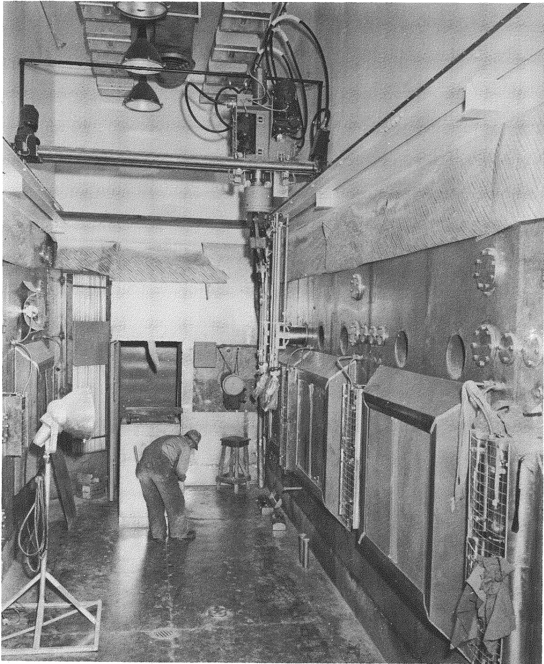
Fig. 19—Interior view of special-services cubicle, ANP, Bldg. 607, Idaho.
