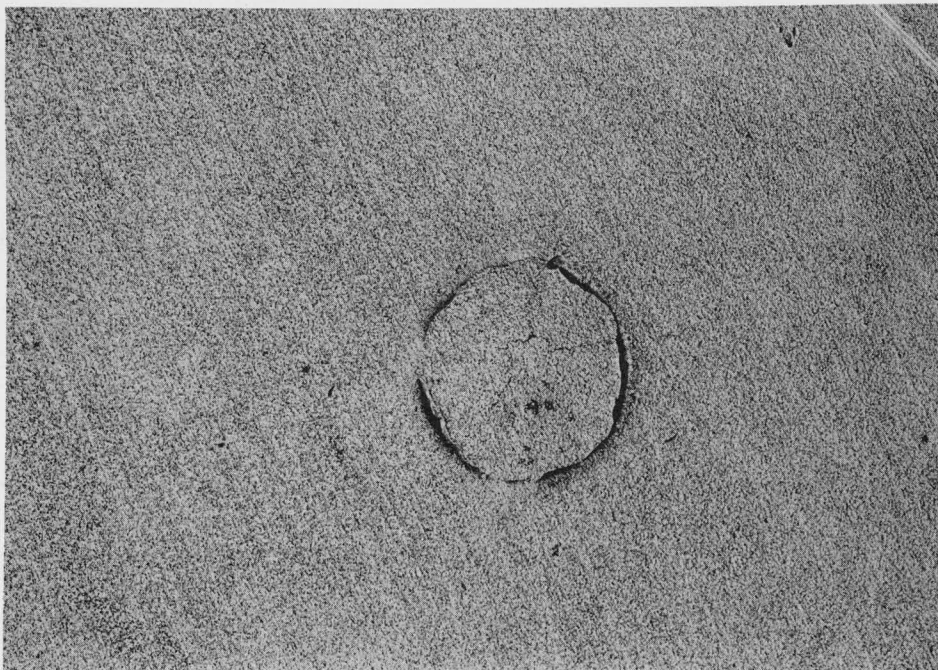
Figure 4. T10154 10X Crack A, see Fig. 2 for location. Water Side of Diaphragm After Scale Removal
