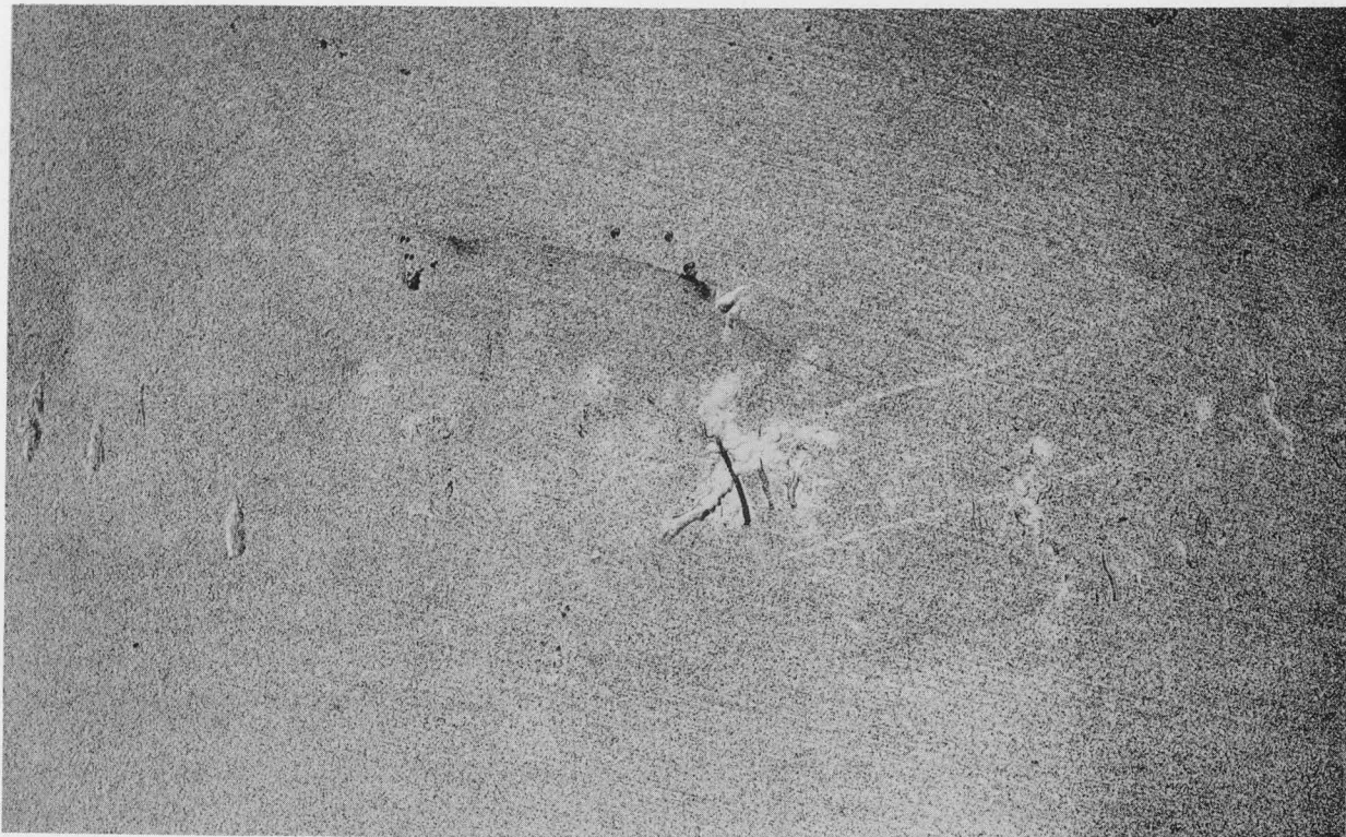
Figure 7 T10162 5X Crack C, See Fig. 1 for Location. Water Side of Diaphragm After Scale Removed
