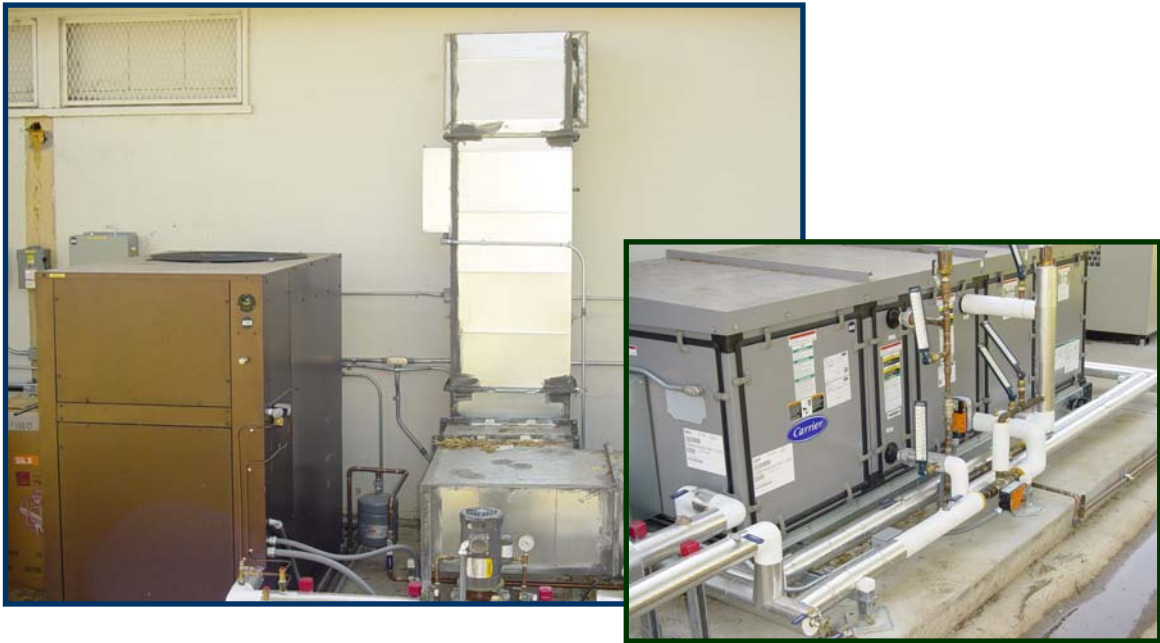
Figure 4. Installation just outside Building C539, NSWC Corona
