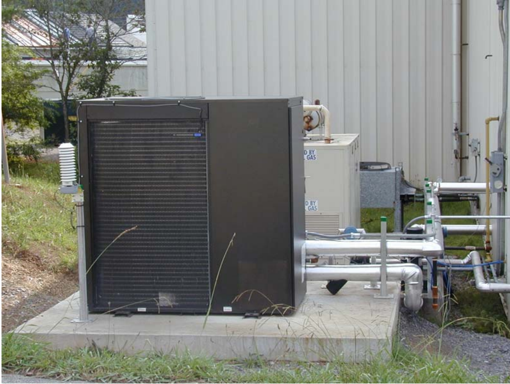
Figure 6. Installation outside Building 3144A, ORNL
