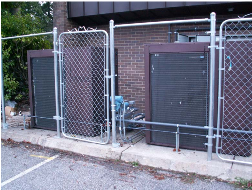
Figure 5. Installation just outside kitchen and laundry area of Building 3364, NAB Little Creek
