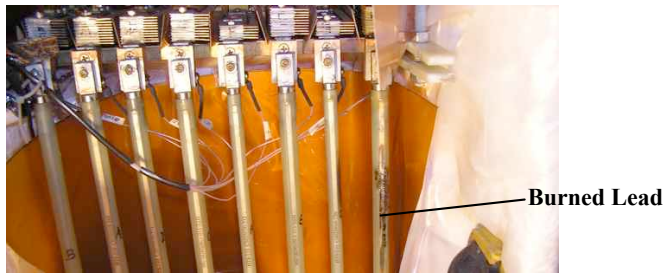
Fig. 6. The HTS leads in Magnet 2 after One Lead Burned Out
