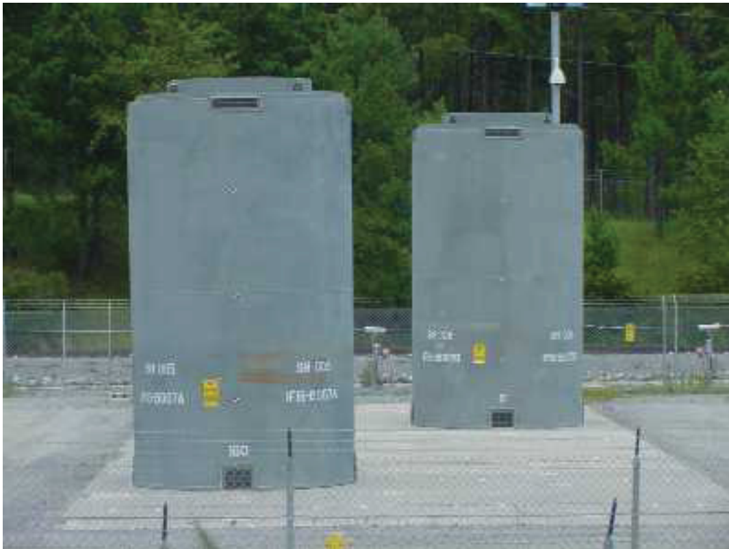
Figure G2-3. Holtec International HI-STORM Dry Storage Casks on storage pad (note vertical storage). Figure taken from Holtec International Web site.
