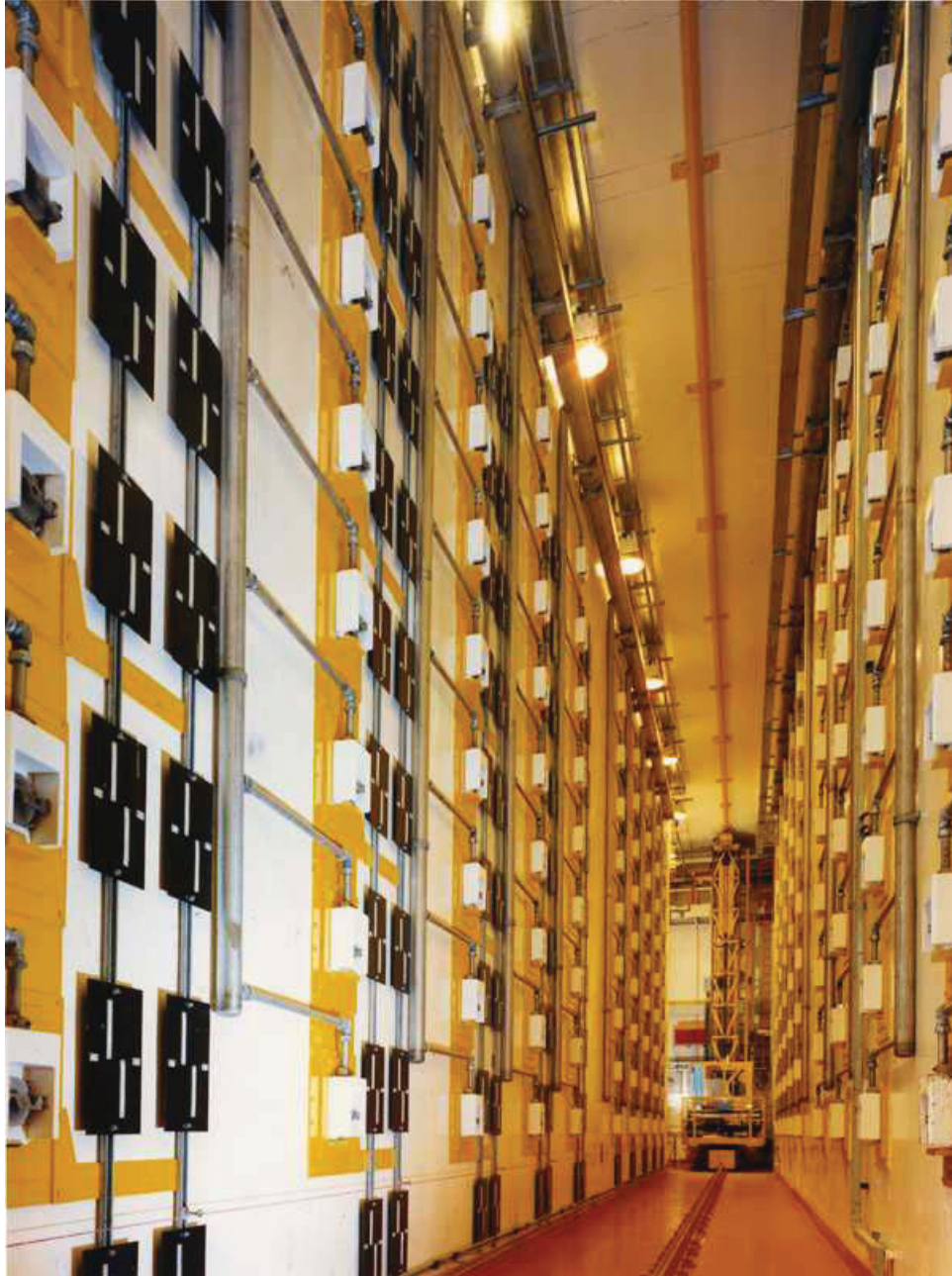
Figure E3-2. Remotely operated store for pure \text{PuO}_2 in welded stainless steel canisters in the THORP facility at Sellafield, U.K.
