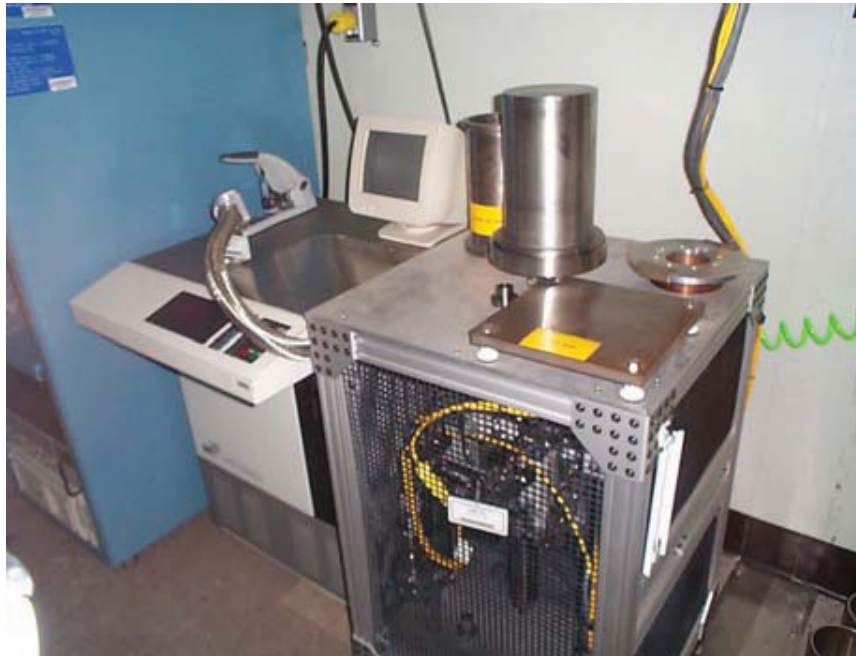
Figure E3-6. Test of leak detector installed in FB-Line Facility at SRS (Hudlow 2004).
