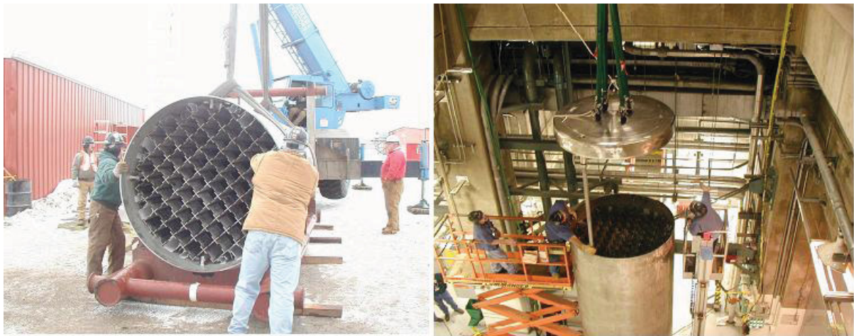
Figure E2-4. Left: Receiving the MPC at J. A. FitzPatrick Nuclear Plant. Right: Fit up of the MPC and MPC lid at J. A. FitzPatrick Nuclear Plant.
