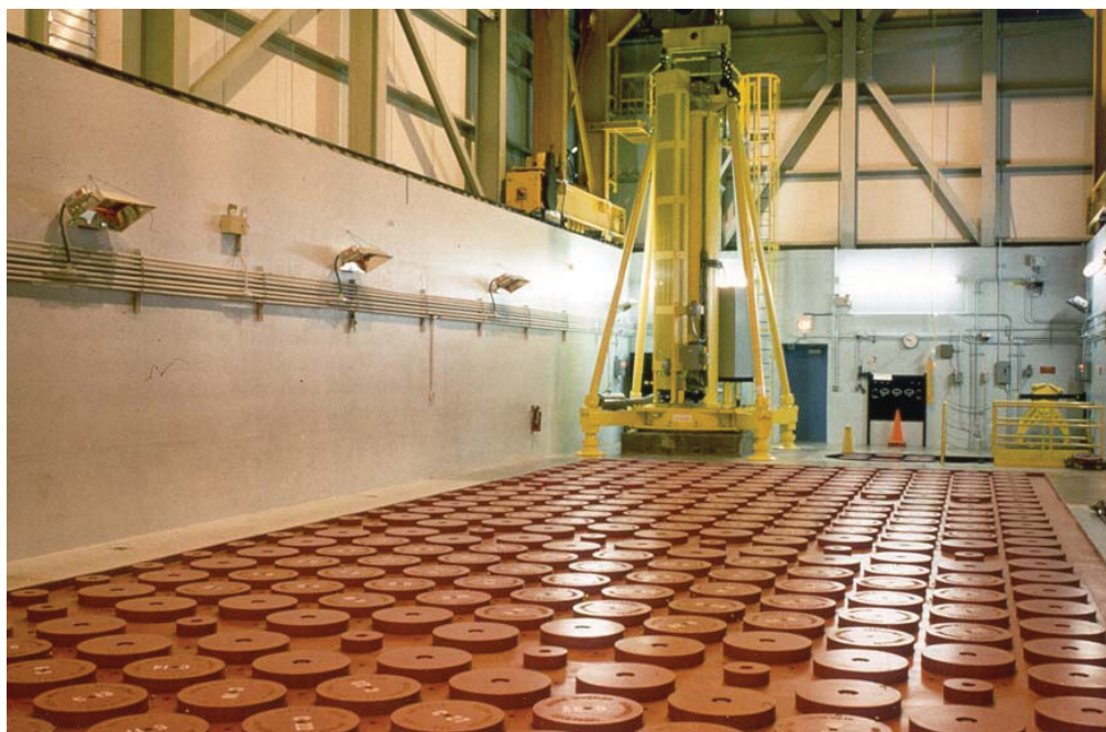
Figure E4-5. Fort St. Vrain modular vault dry store (MVDS) showing charge face.
