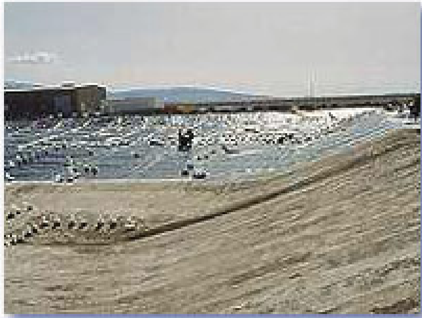
Figure G3-4. Landfill disposal cell at EnergySolutions (Note line and leachate collection piping). Figure taken from EnergySolutions Web site.
