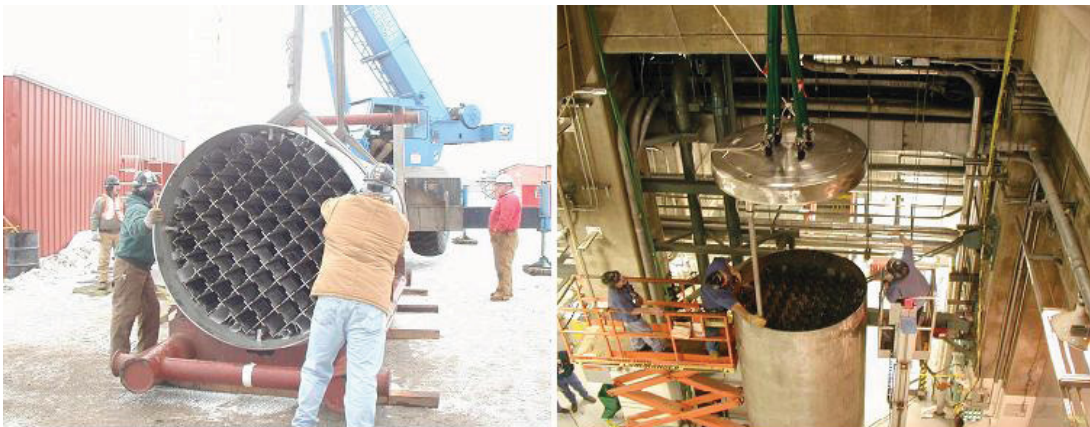
Receiving the MPC at J.A. FitzPatrick Nuclear Plant
