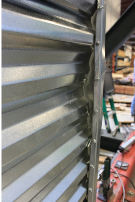
(a) Screw shear failure
