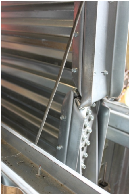
(c) Chord framing member buckles
