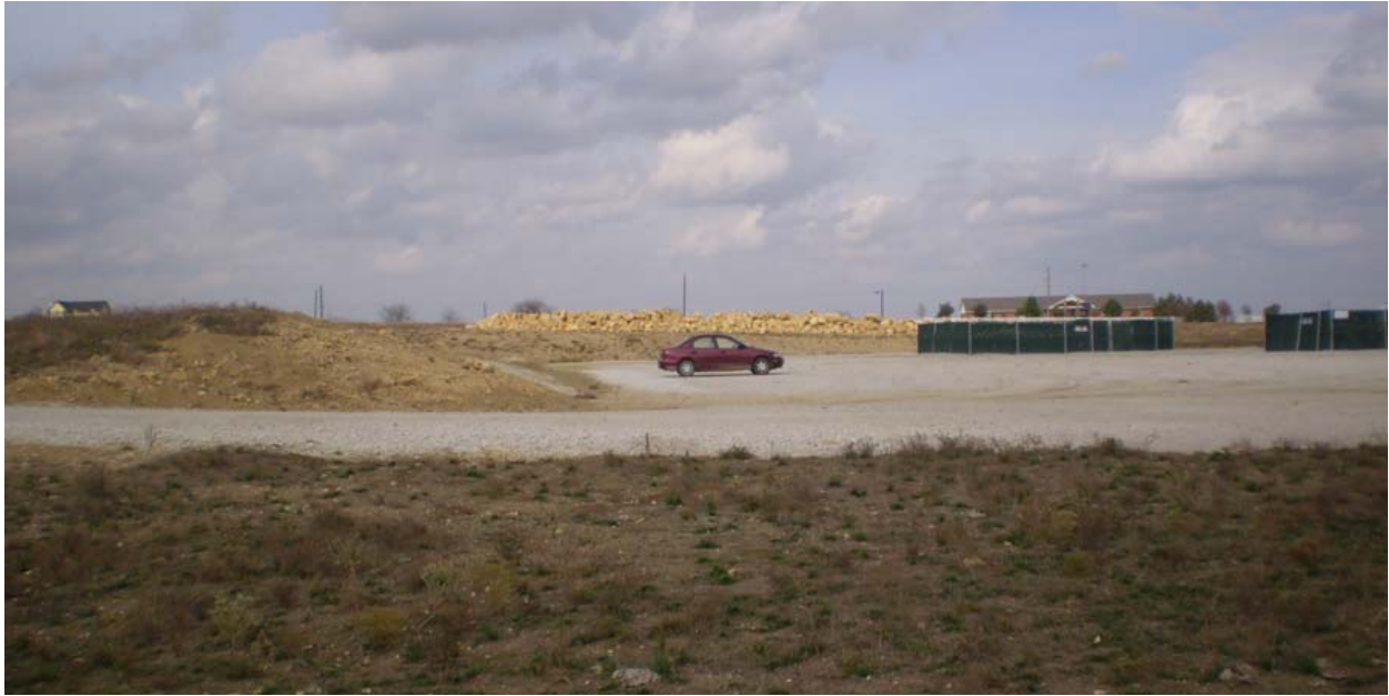
Figure 5. Gas well pad cut into hillside. Original hill slope slants from left to right behind the car and, where the car is parked, has been cut away by six or more feet to create the flat pad area.
