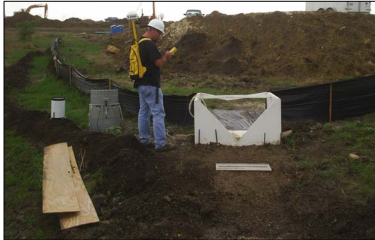
Figure 9. Weir setup. A slotted sediment trap is installed a few feet in front of this weir. Plywood pieces were later attached to the weir to make a channel directing water over the trap. Erosion between the weir and trap was prevented by lining the channel with heavy plastic.
