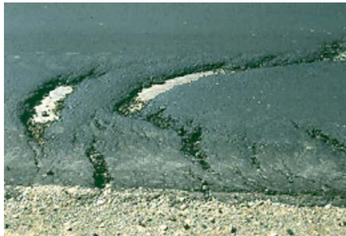
Figure 7: Slippage cracks Courtesy: Kearney et al. 2004
