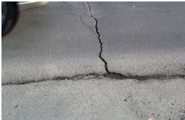
Figure 4: Transverse crack Courtesy: Kearney et al. 2004
