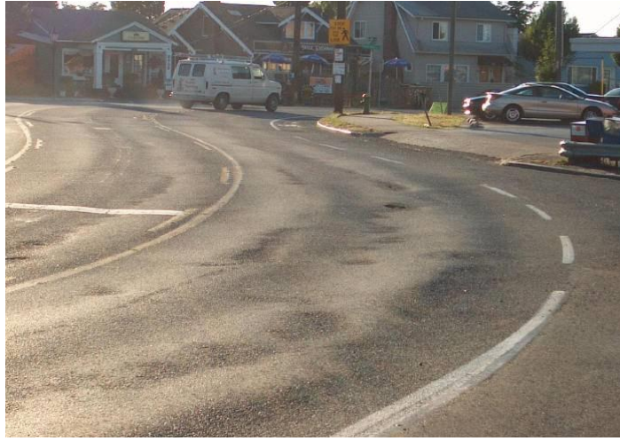
Figure 8: Rutting Courtesy: Donald et al. 1987, 1989, 2002
