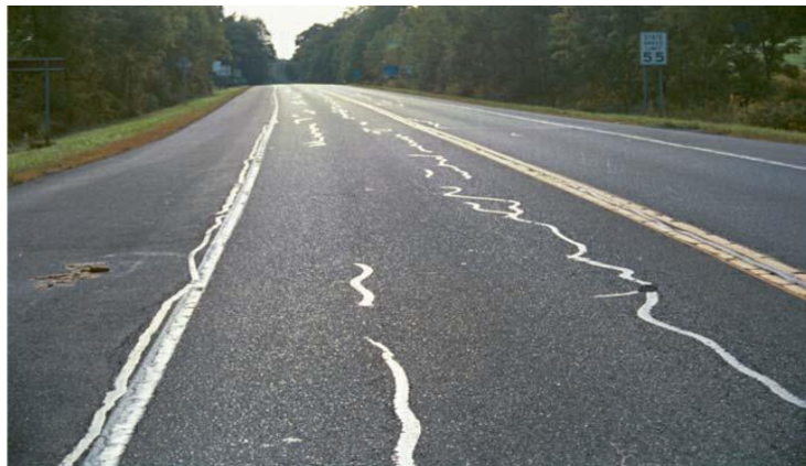
Figure 6: Longitudinal wheel path cracking Courtesy: Kearney et al. 2004
