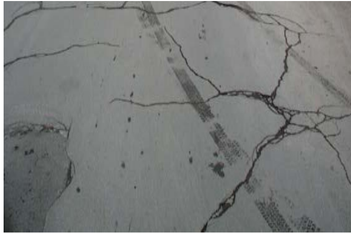
Figure 5: Block cracking Courtesy: Kearney et al. 2004
