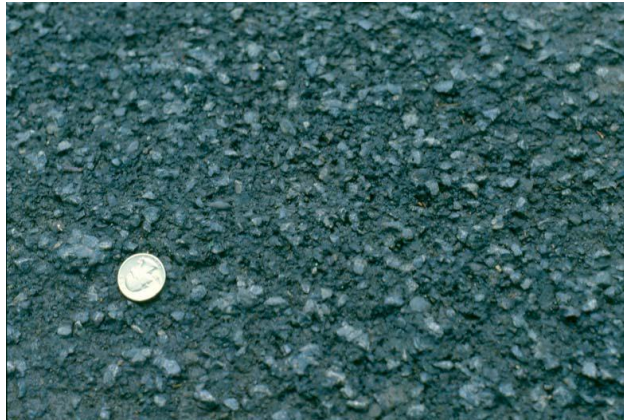
Figure 11: Surface raveling of an asphalt pavement Courtesy: Kearney et al. 2004
