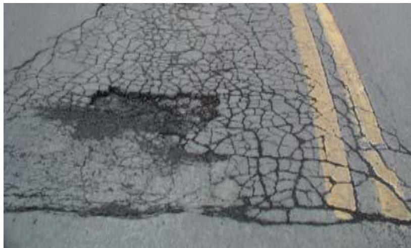
Figure 3: Alligator cracks with pothole Courtesy: Kearney et al. 2004
