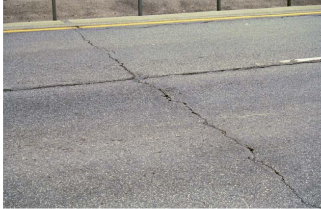
Figure 2: Reflective cracks Courtesy: Kearney et al. 2004
