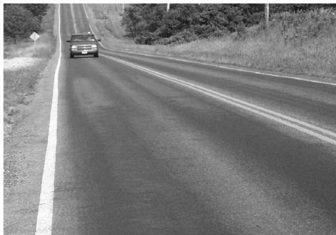
Figure 12: Bleeding asphalt Courtesy: Kearney et al. 2004
