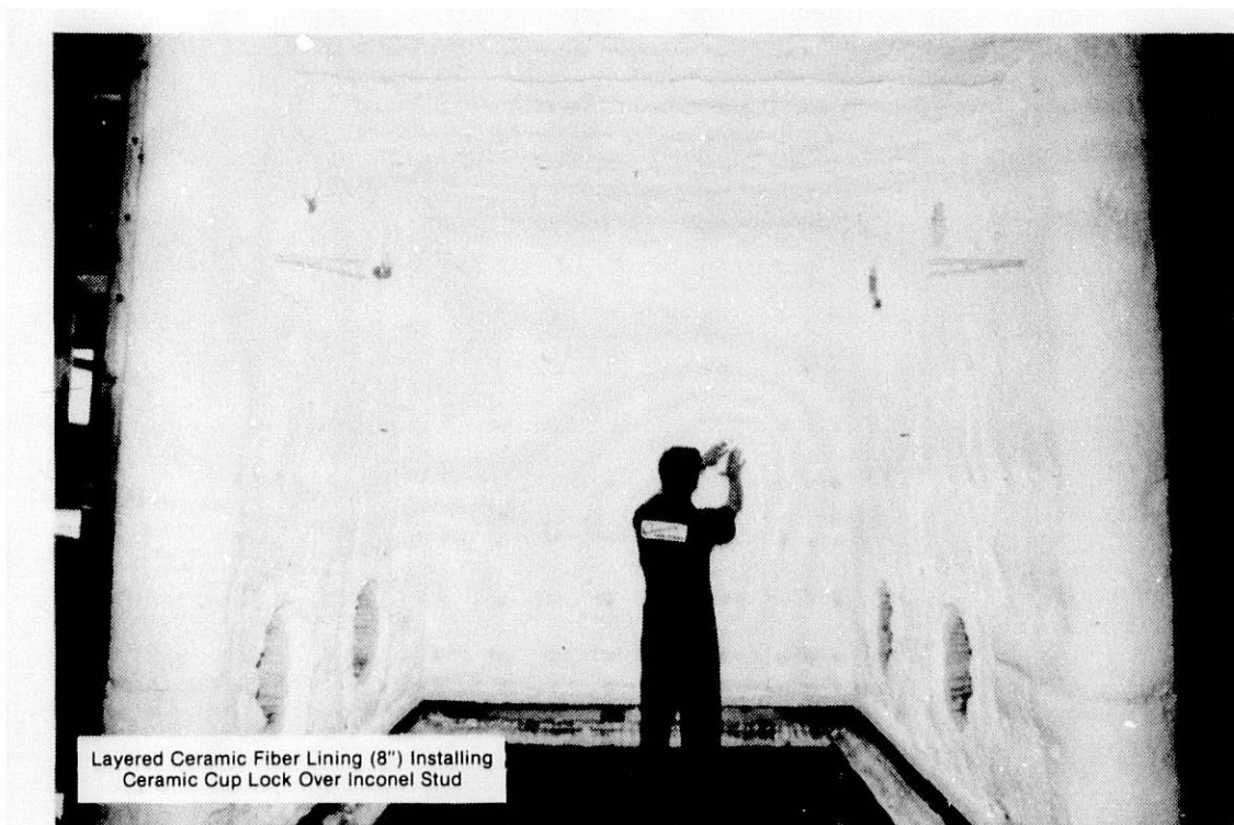
Fig. 2. Large industrial furnace refitted with ceramic fiber layered insulation. Fuel savings over 50% relative to hard brick insulation. (Photograph courtesy of Gas Research Institute, Chicago, IL).
